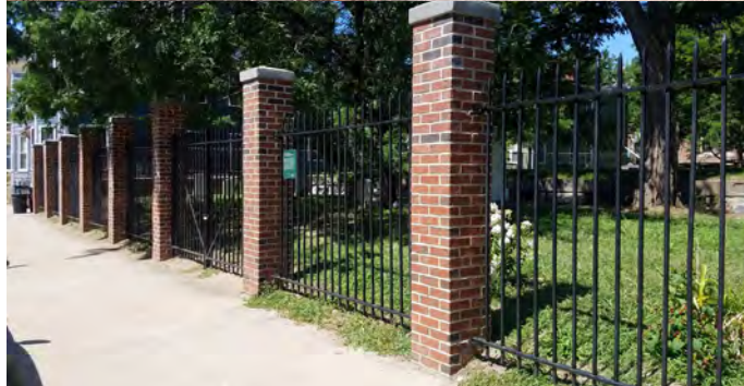
Above: Crumbling bricks at the bottom of the pier contributed to structural instability. Below: The finished product. The same brick was used for all of the piers creating a uniform look.
