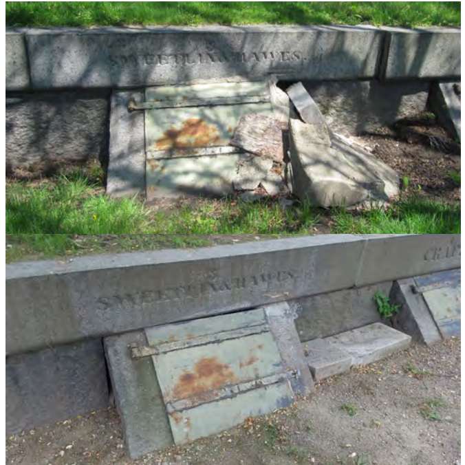
Before and after photos of the repair of the broken tomb doorway.
