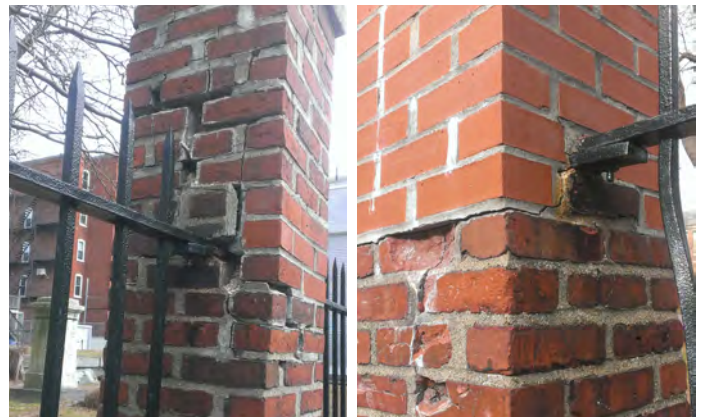
These close-up shots of two different columns illustrate some of the problems. The left column shows extensive cracking and mortar loss. The right column shows more cracking and two types of bricks.
