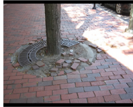
The once beautiful brick sidewalks pose a safety hazard to pedestrians and are in dire need of repair.
