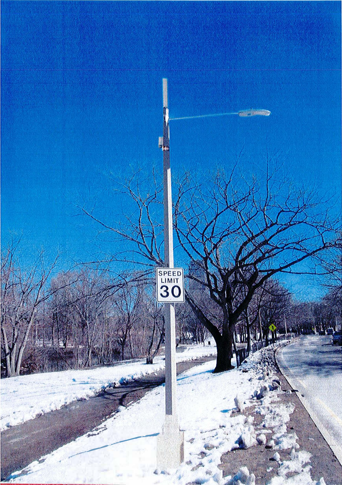
Example of standard steel light pole with approved wireless facility installed
