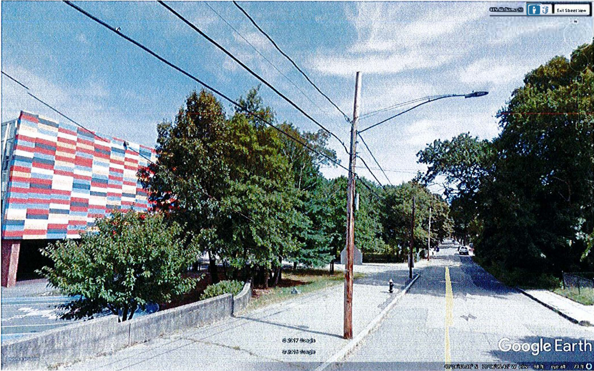
Example of wood utility pole (top mount)
