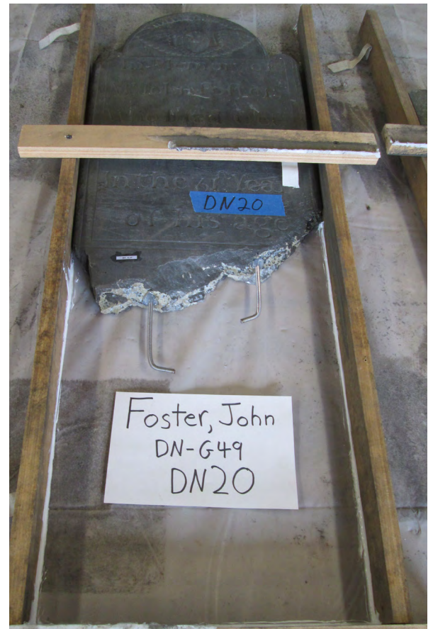
The John Foster headstone during restoration. The pins have been installed and the form for the concrete base has been built.
