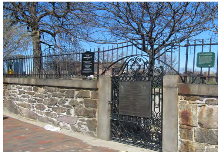
The iron fence on top of the puddingstone wall is being restored.
