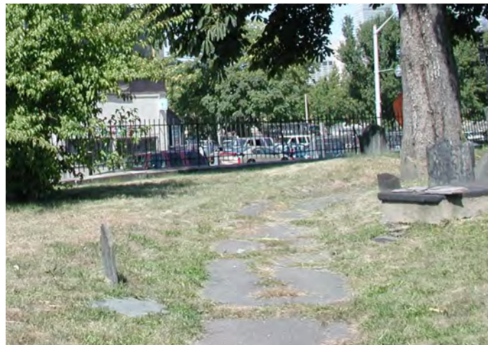
The old asphalt pathway had many cracks. Grass was growing through the cracks and encroaching on the edges.
