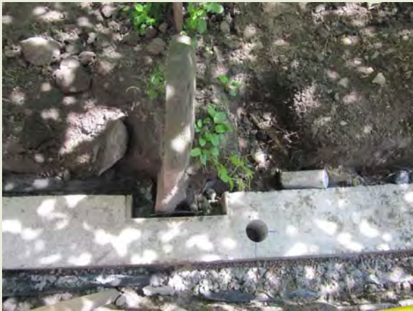
A cut-out is made in the concrete grade beam to accommodate a headstone.
