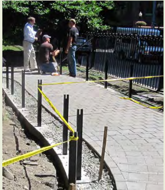
A section of widened pathway with fence posts set in the exposed concrete grade beam.
