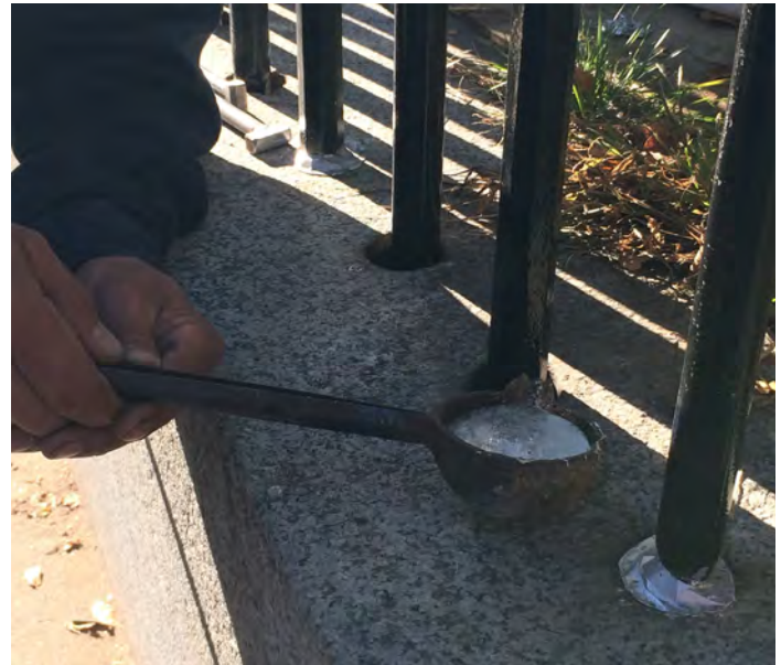
Molten lead is being poured into the picket hole by the contractor.
