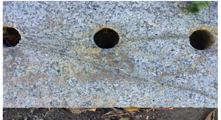
The crack repairs on the top of the wall closely match the granite.
