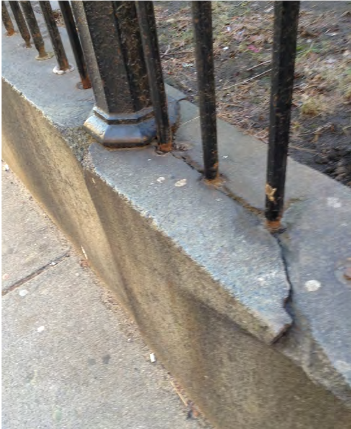
Before restoration there were many cracks in the top of the granite wall. Every winter the freeze and thaw cycles makes the cracks larger.
