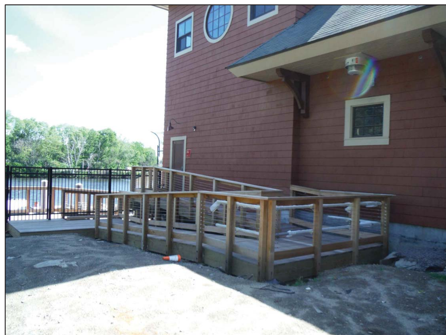
D PHOTO D - EXISTING RAMP RAILINGS NOT TO SCALE
