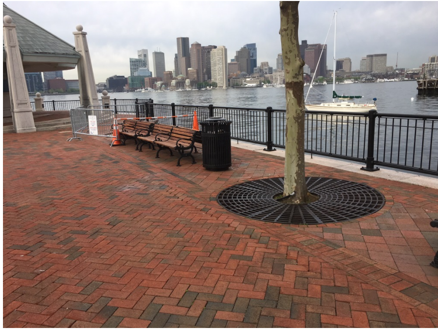
Photo 3: Area of Sinkhole
