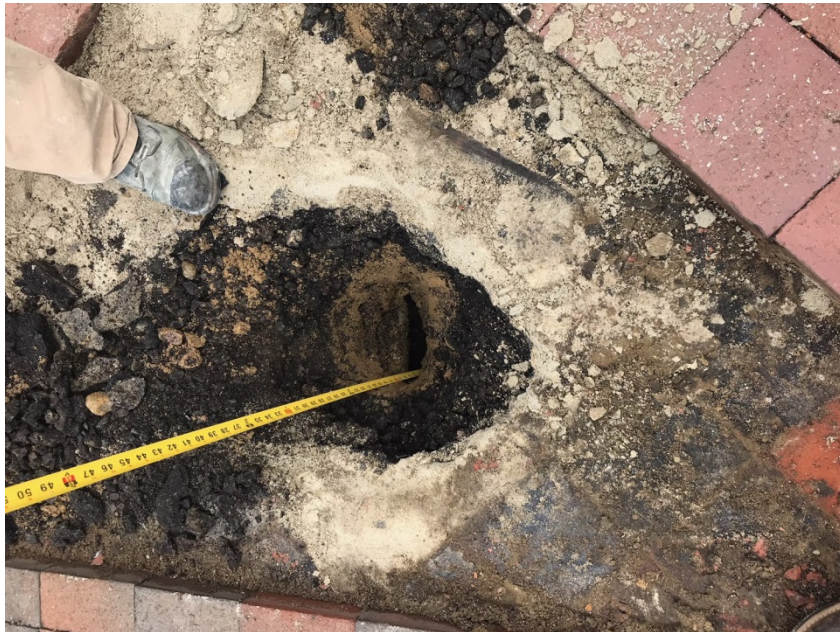
Photo 4: Sinkhole is several feet deep and currently undermines a section of walkway.
