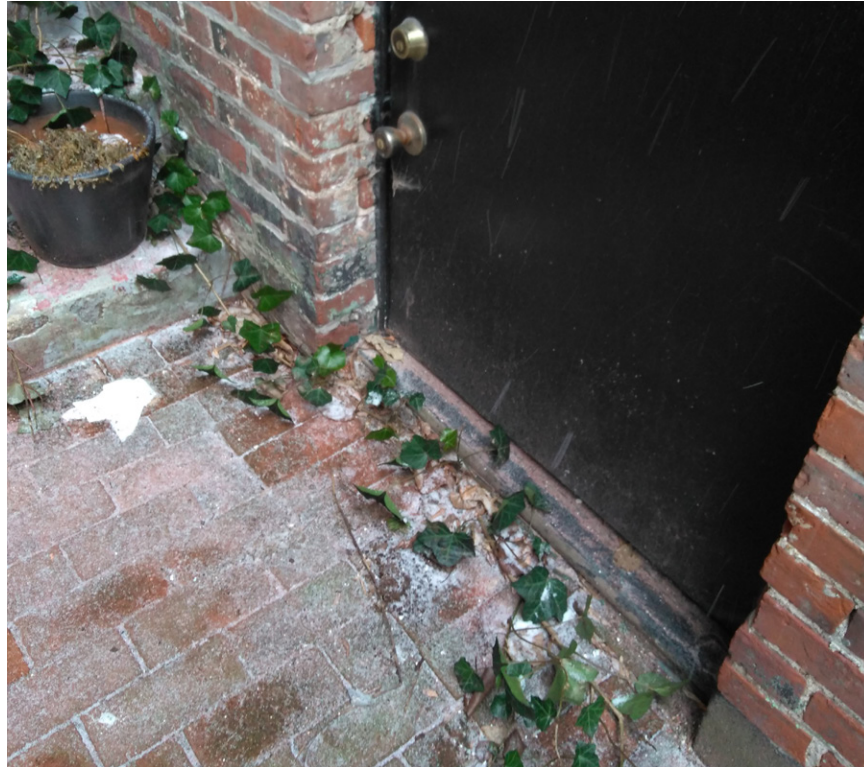
⑥. PROPER FUNCTION OF EMERGENCY EGRESS DOOR
