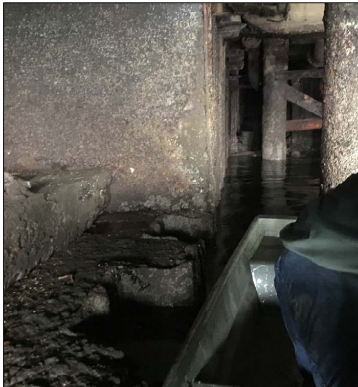
Photo No. 20: Floor of the discharge end of the culvert. Note the sheet pile wall along the underside of the culvert.
