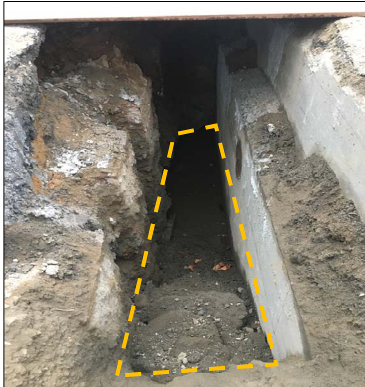
Photo No. 5: 3-foot thick concrete plug placed between the concrete wall and the steel sheet pile wall before backfilling.
