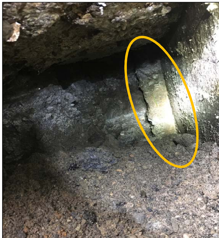
Photo No. 4: View of the void below the concrete plug. A concrete seal appears to be at the intersection of the SSP and the concrete culvert wall.
