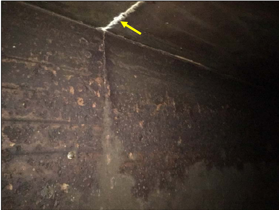
Photo No. 13: Typical wall and ceiling joint intersection. Note efflorescence along roof joint.
