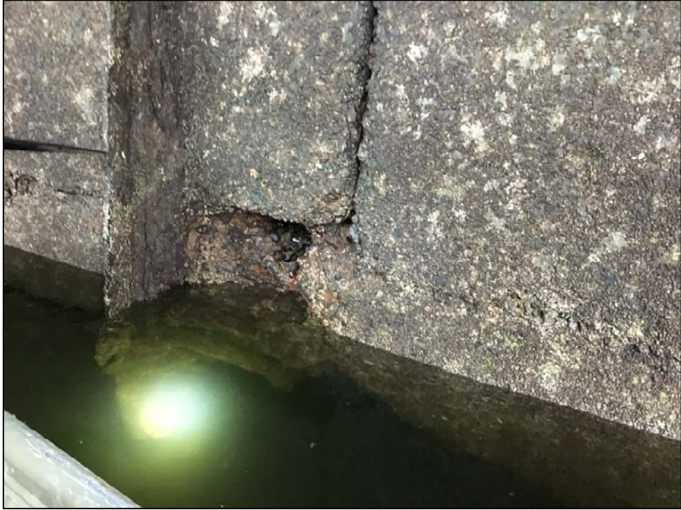
Photo No. 21: View of the cut sheet pile wall from the outside of the culvert, approximately 50 feet from the discharge end.
