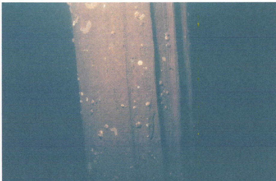
Photo #2 showing intact pile with deep striations
