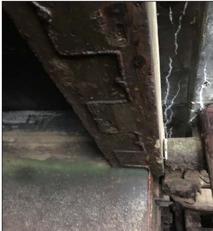
Photo No. 19: Discharge end of the culvert ceiling. Note the culvert appears to protrude through a sheet pile wall.
