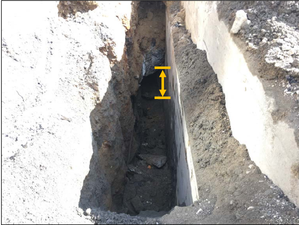
Photo No. 3: Overview of TP1 after the excavation was complete. Note the void below the concrete plug.
