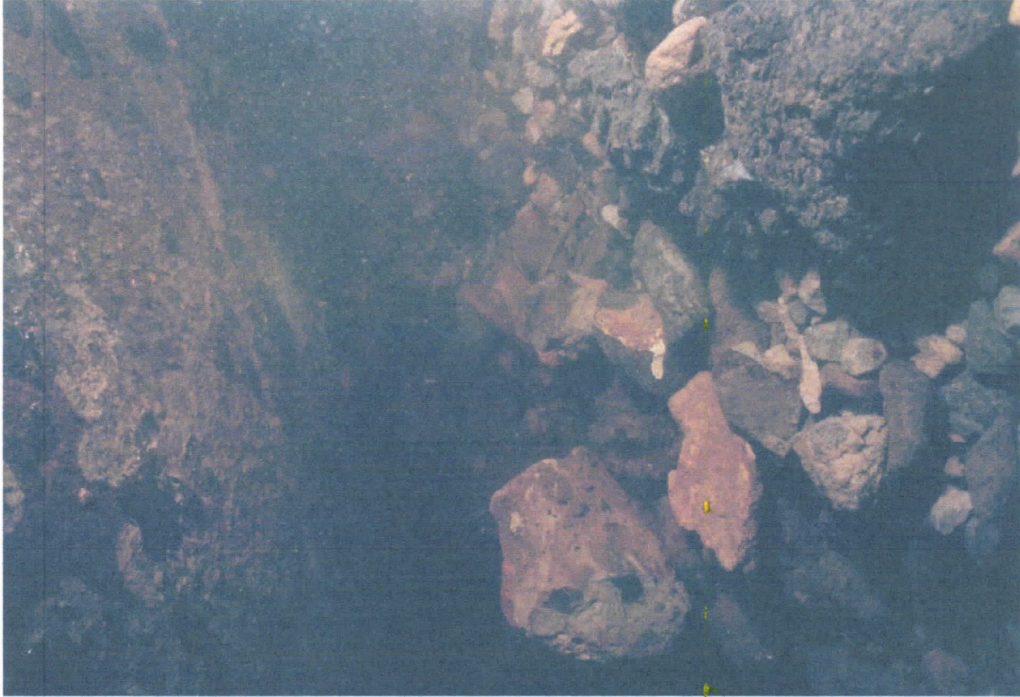
Photo #3 showing typical rubble fill between the sheet pile wall and the culvert wall
