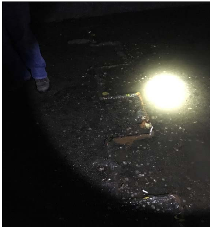
Photo No. 16: Sheet pile wall protruding through the floor of the culvert, approximately 50 feet from the discharge end of the culvert.
