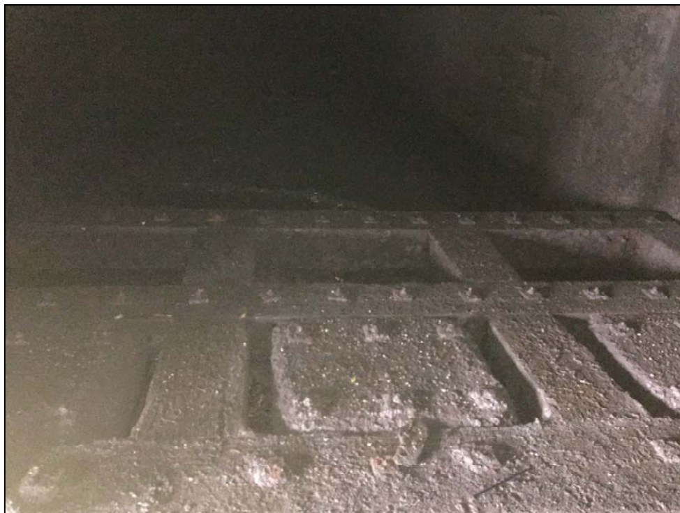
Photo No. 10: Overview of the tide gate on the floor of the culvert. Note the gate is no longer operational.
