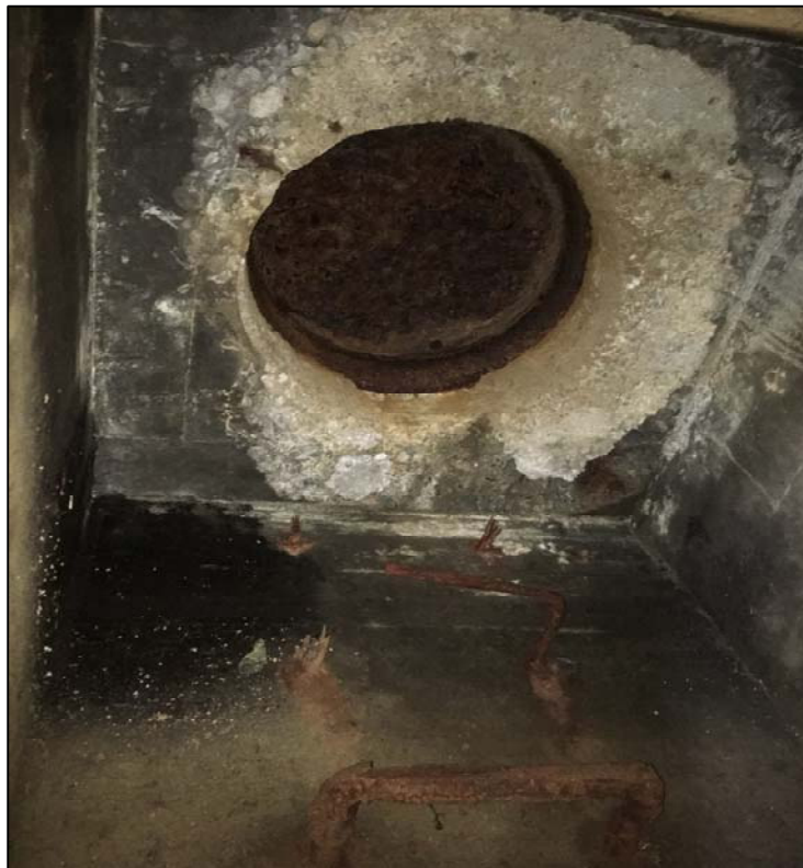
Photo No. 18: Access to culvert hatch opening. Access is not visible from the topside and appears to be abandoned.
