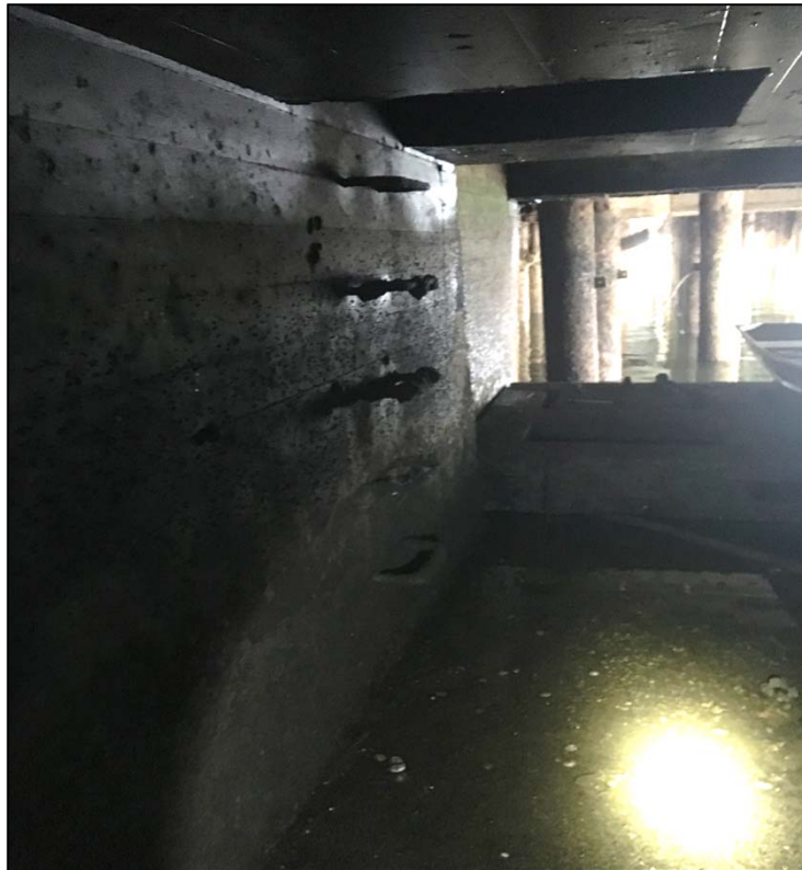
Photo No. 17: Culvert access ladder approximately 15 feet from the discharge end of the culvert.
