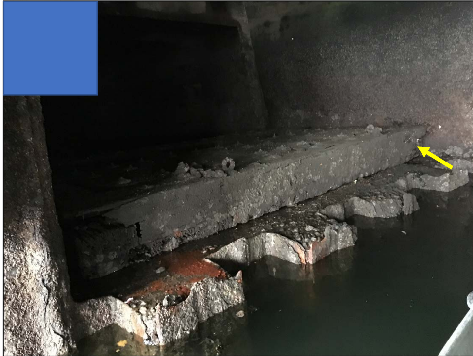
Photo No. 9: View of the discharge end of the culvert. The tide gate is laying at the bottom of the culvert and detached from its hinges.
