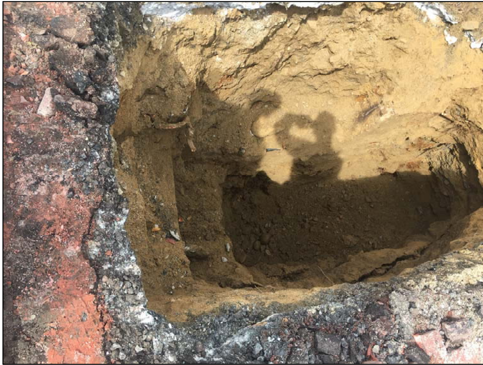
Photo No. 7: Overview of TP2, note the soil appears to be dry intact.
