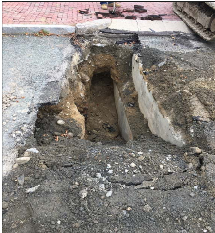
Photo No. 2: Overview of Test Pit 1 (TP1). The excavation is approximately 50% completed within this picture.
