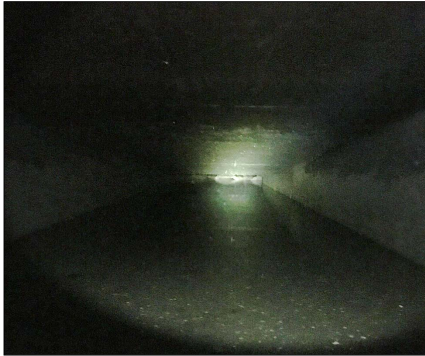
Photo No. 15: Overview of the inside of the culvert looking towards the pump house and the 45-degree bend.
