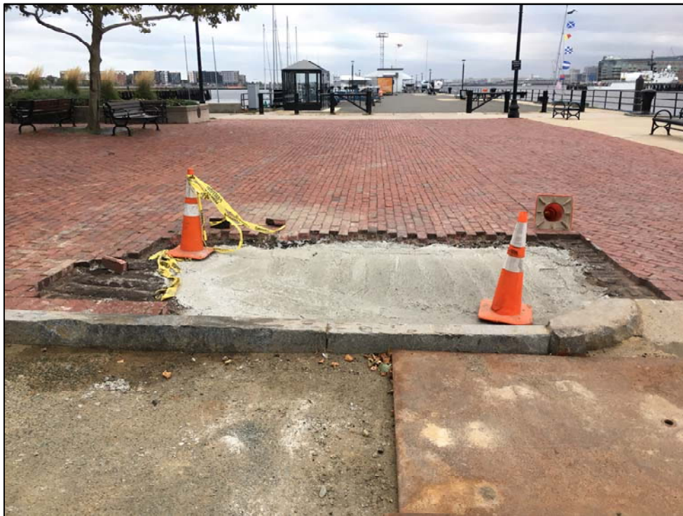
Photo No. 8: Overview of TP2 after it was backfilled. A concrete overlay was placed at the top of the test pit.
