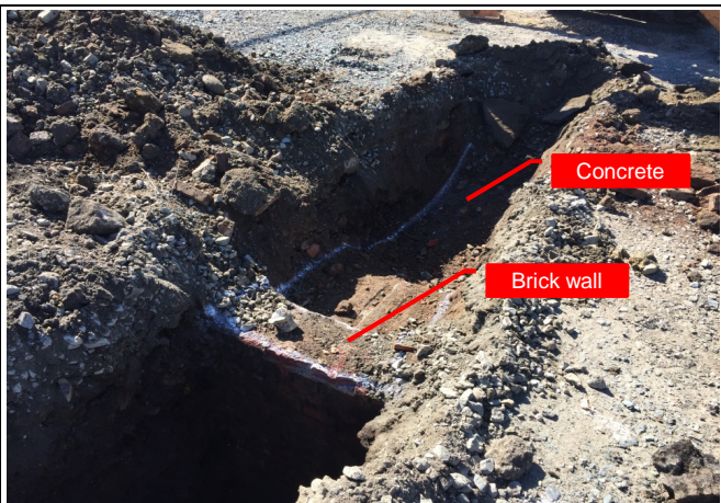
Photo 3 - Excavation refusal in western half of test pit on buried concrete (possible concrete slab).
