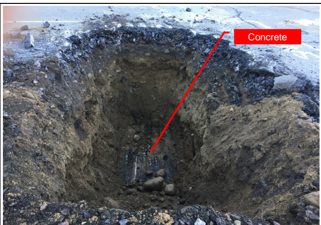
Photo 3 - Excavation refusal on buried concrete (possible concrete slab).
