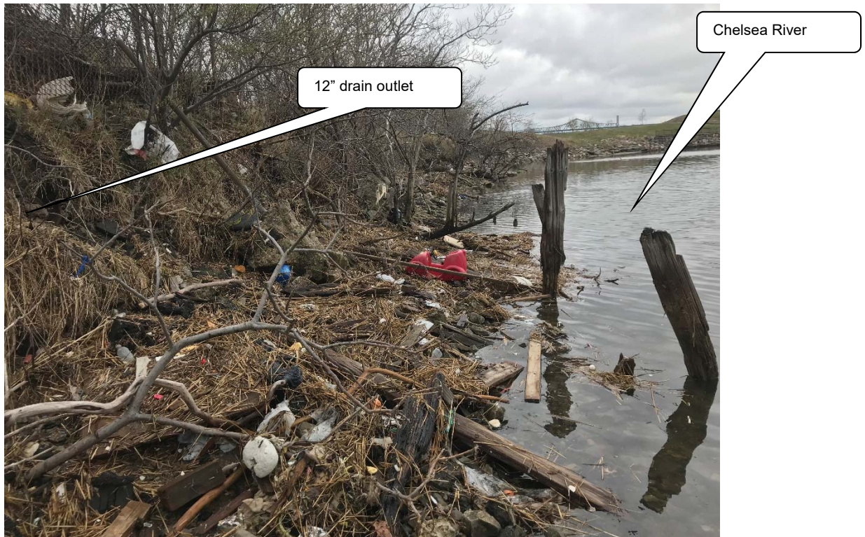
Photo 6 – Existing 12" drain outlet into Chelsea River
