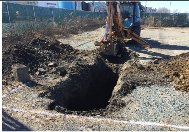
Photo 1 - Looking west at test pit location. Test pit located immediately west of paved access road in gravel area.
