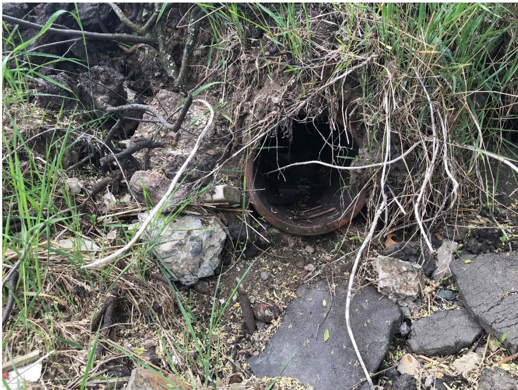
Photo 8 – Existing 12" drain outlet into Chelsea River
