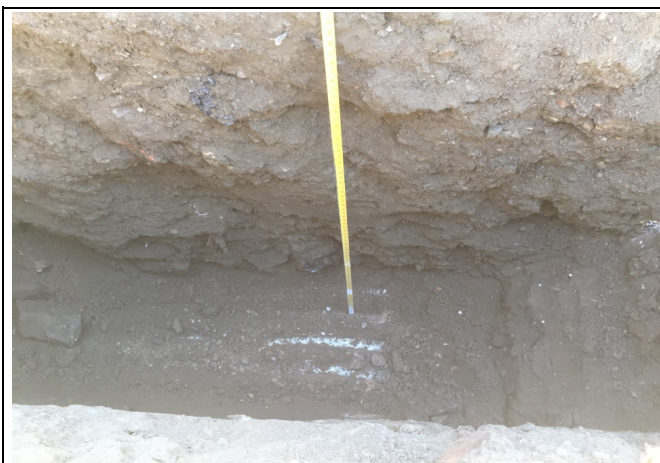
Photo 5 - Excavation refusal on buried concrete (possible concrete slab).
