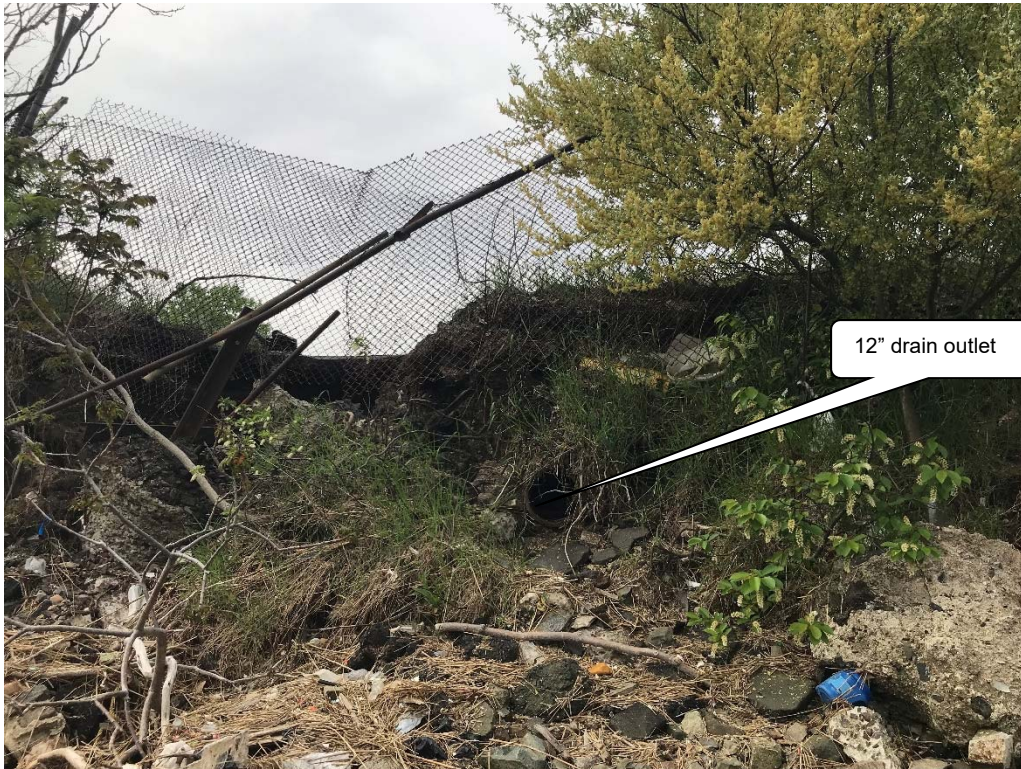
Photo 7 – Existing 12" drain outlet into Chelsea River
