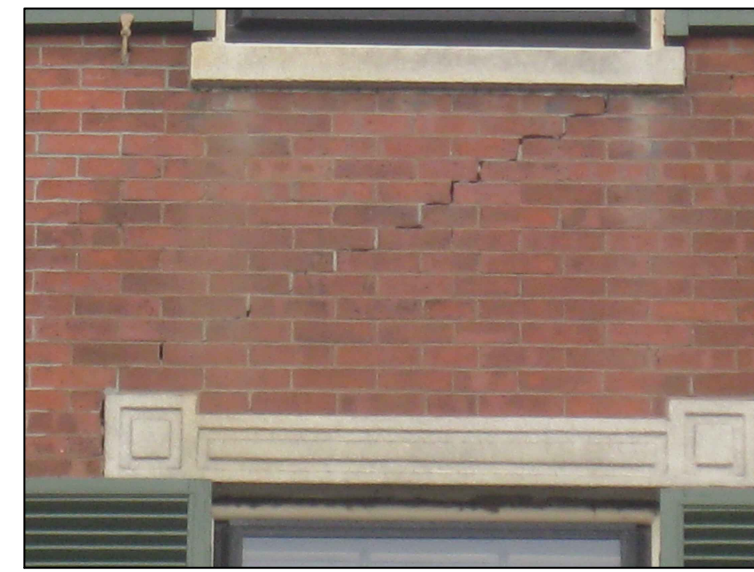
SOUTH ELEVATION STEP CRACK 18 EXISTING CONDITIONS - PHOTO 18 SCALE: NOT TO SCALE
