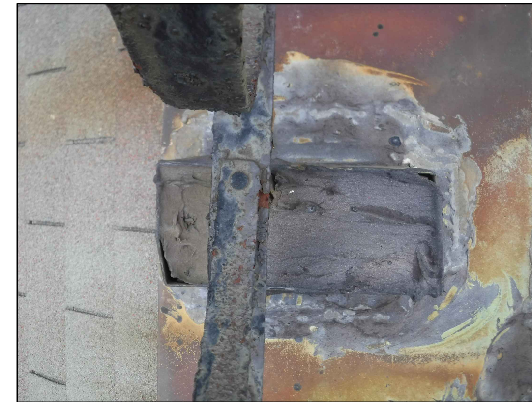
VIEW OF LOOKING DOWN AT RAILING SUPPORT 30 EXISTING CONDITIONS - PHOTO 30 SCALE: NOT TO SCALE
