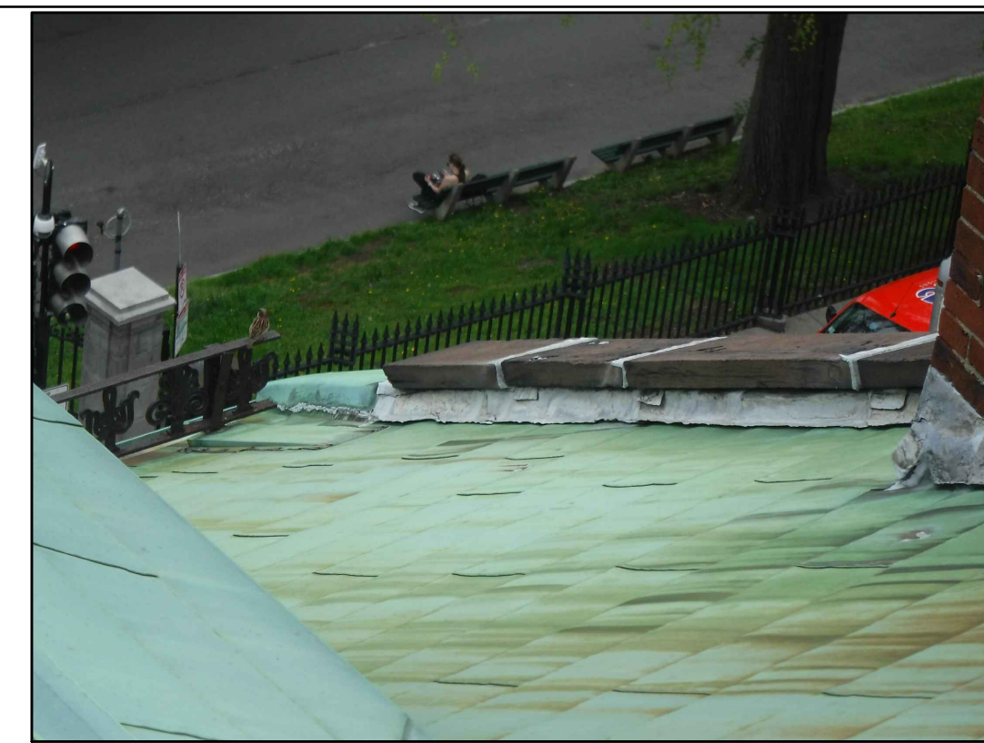
PARTY WALL AT SOUTH WEST CORNER OF ROOF 6 EXISTING CONDITIONS - PHOTO 6 SCALE: NOT TO SCALE
