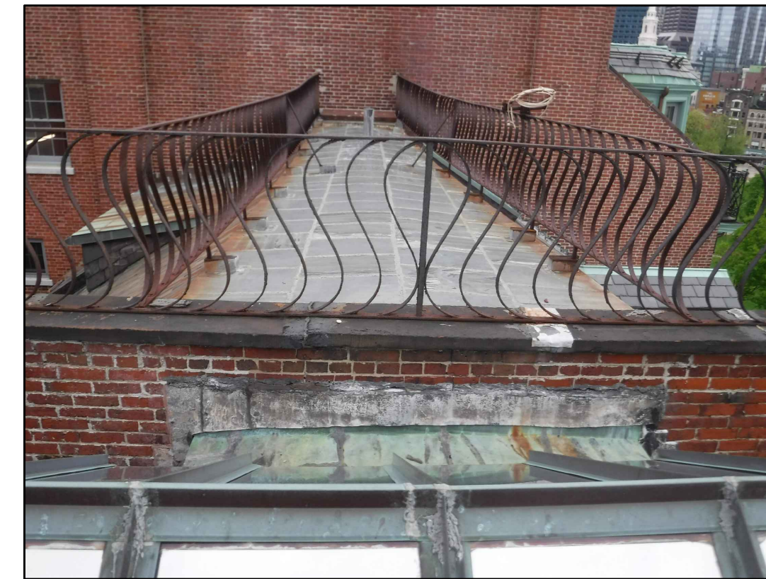
FLASHING AT EAST PARAPET RIDGE 29 EXISTING CONDITIONS - PHOTO 29 SCALE: NOT TO SCALE
