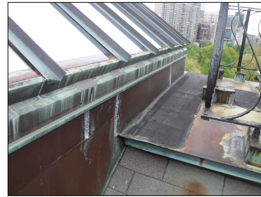
SKYLIGHT AND EAST END OF FLAT ROOF 21 EXISTING CONDITIONS - PHOTO 21 SCALE: NOT TO SCALE
