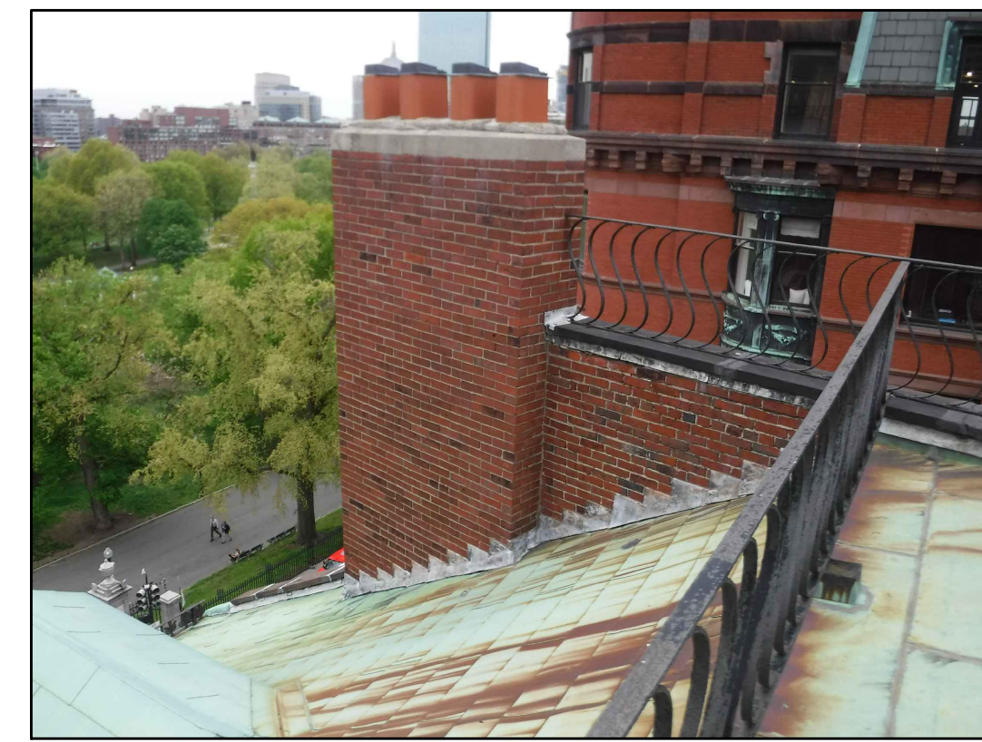
WEST PARAPET AT SOUTH ROOF 11 EXISTING CONDITIONS - PHOTO 11 SCALE: NOT TO SCALE
