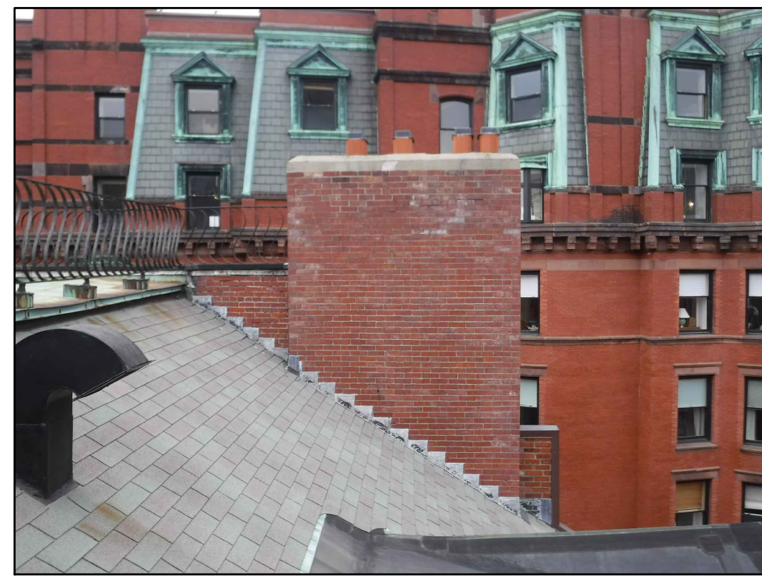
WEST VIEW OF NORTH ROOF 7 EXISTING CONDITIONS - PHOTO 7 SCALE: NOT TO SCALE
