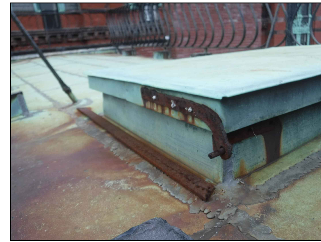
ROOF HATCH ON FLAT ROOF 24 EXISTING CONDITIONS - PHOTO 24 SCALE: NOT TO SCALE
