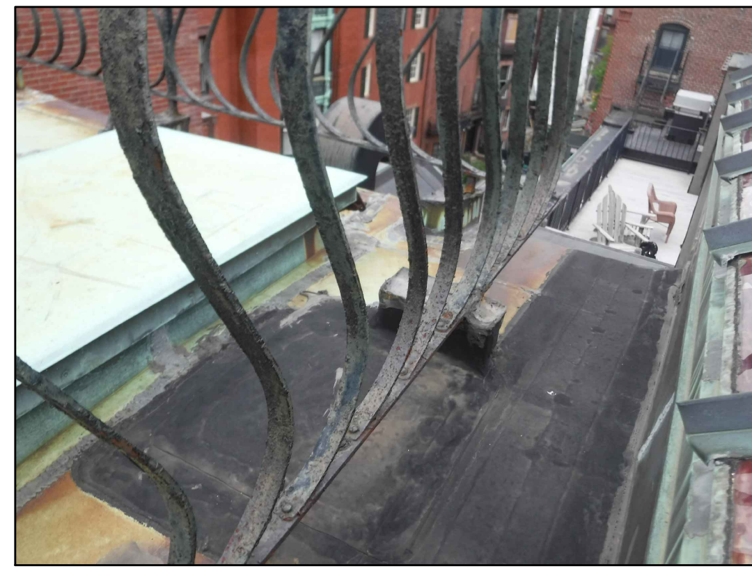
EAST END OF FLAT ROOF 20 EXISTING CONDITIONS - PHOTO 20 SCALE: NOT TO SCALE
