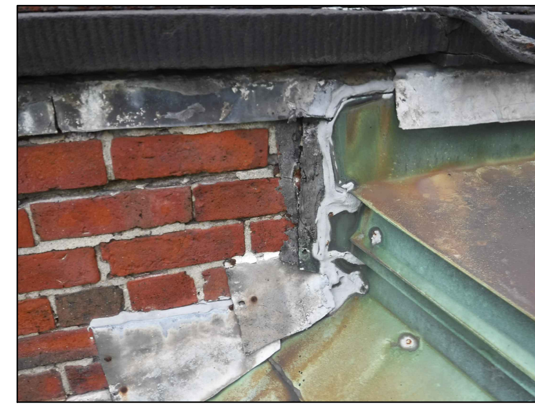
FLASHING AT WEST PARAPET SOUTH ROOF 12 EXISTING CONDITIONS - PHOTO 12 SCALE: NOT TO SCALE
