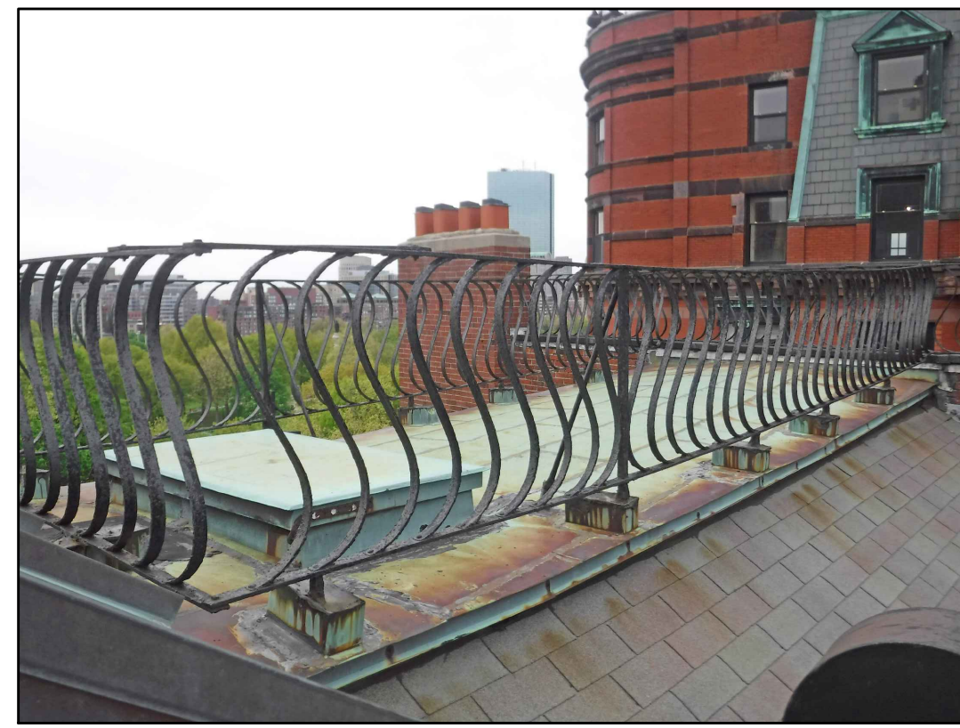
NORTH WEST VIEW OF FLAT ROOF 19 EXISTING CONDITIONS - PHOTO 19 SCALE: NOT TO SCALE
