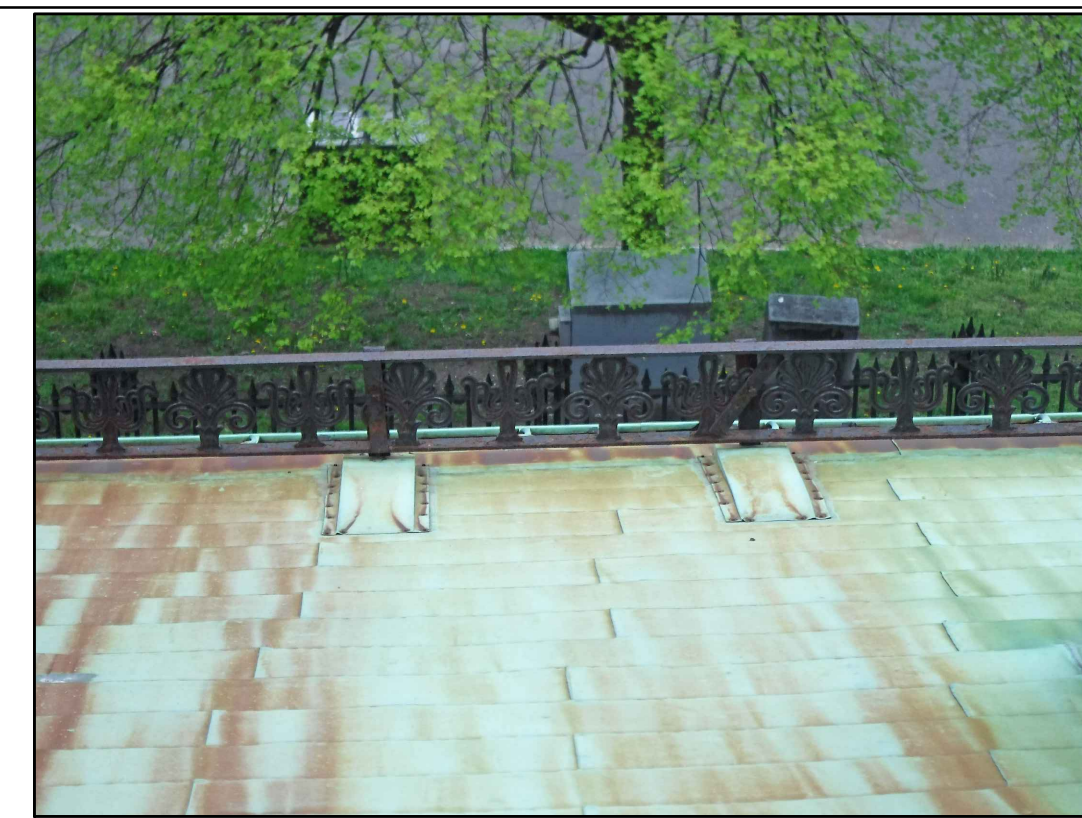
VIEW OF SOUTH ROOF ORNAMENTAL EDGE 5 EXISTING CONDITIONS - PHOTO 5 SCALE: NOT TO SCALE
