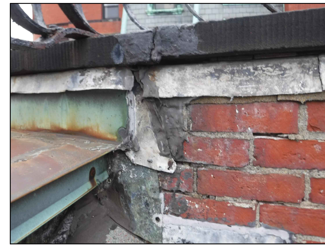
WEST PARAPET WALL FLASHING AT NORTH ROOF 10 EXISTING CONDITIONS - PHOTO 10 SCALE: NOT TO SCALE
