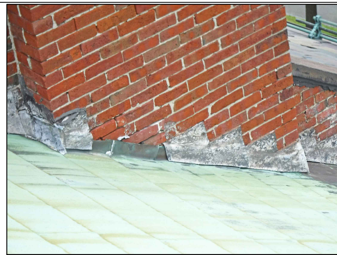
FLASHING AT SOUTH EAST CHIMNEY 2 EXISTING CONDITIONS - PHOTO 2 SCALE: NOT TO SCALE
