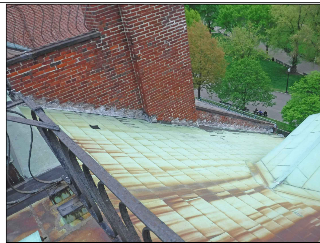
VIEW OF SOUTH EAST ROOF 1 EXISTING CONDITIONS - PHOTO 1 SCALE: NOT TO SCALE
