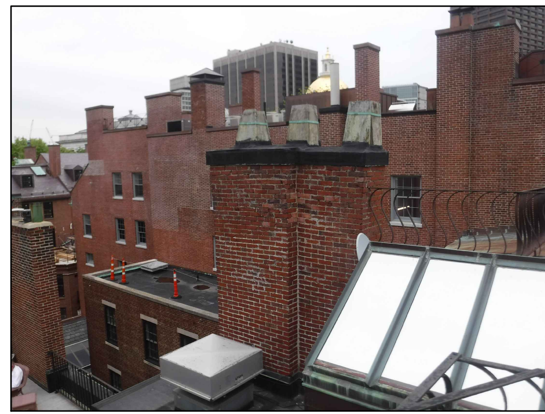
VIEW OF NORTH EAST CHIMNEY 14 EXISTING CONDITIONS - PHOTO 14 SCALE: NOT TO SCALE
