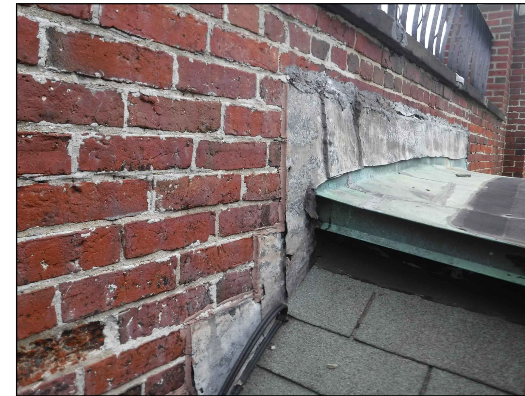
NORTH ROOF RIDGE AND EAST PARAPET 28 EXISTING CONDITIONS - PHOTO 28 SCALE: NOT TO SCALE
