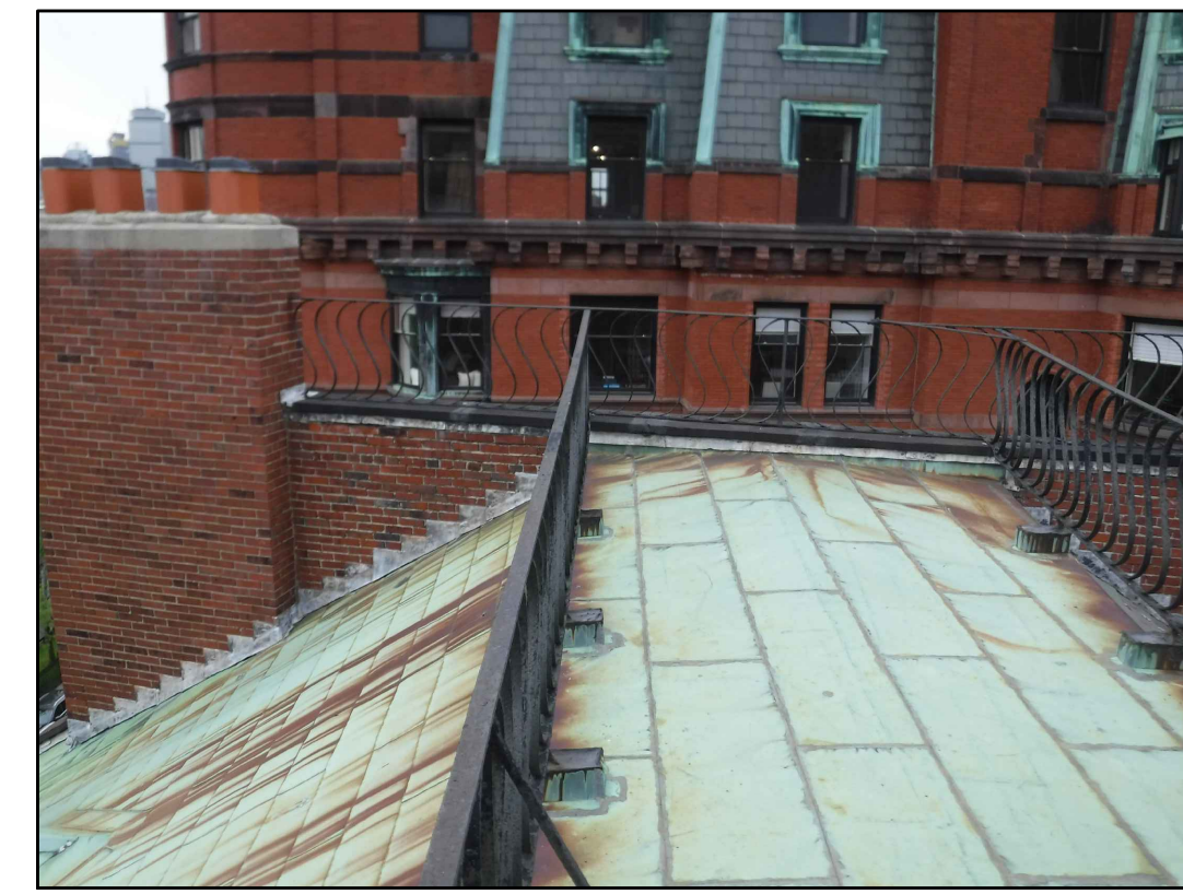
EAST END OF FLAT ROOF 23 EXISTING CONDITIONS - PHOTO 23 SCALE: NOT TO SCALE
