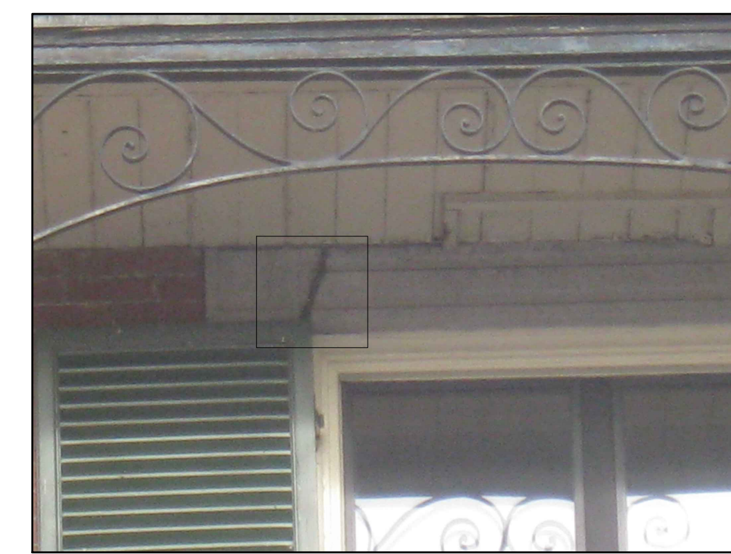
A EXISTING CONDITIONS - PHOTO 1 NOT TO SCALE
