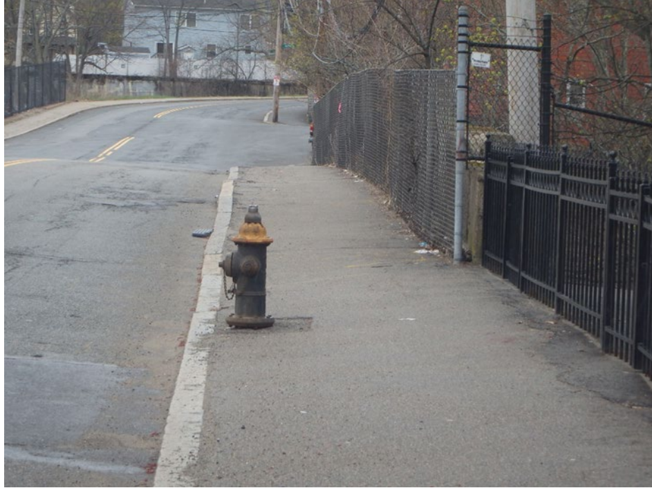
Photo 3: North approach looking at west sidewalk along Dana Avenue, Hyde Park, Boston, MA.
