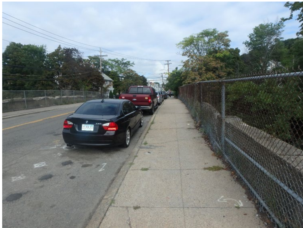
Photo 6: South approach looking at east sidewalk along Dana Avenue, Hyde Park, Boston, MA.
