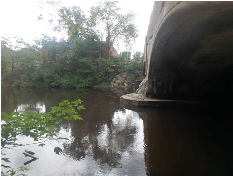
Photo 10: North end looking at downstream bank along Neponset River, Hyde Park, Boston, MA.
