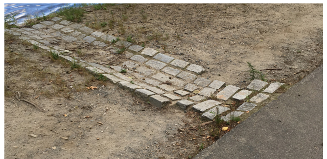
Example of cobblestone spillway that will be repaired and retrofit with a sediment trap inlet.
