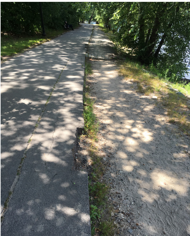
Compaction and erosion leaves bituminous pavement several inches higher than the adjacent surface.
