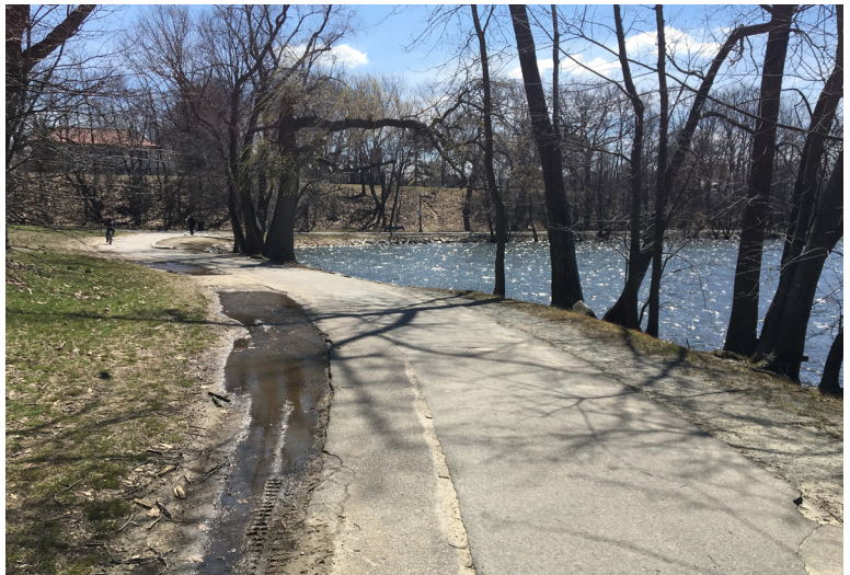
Pathway alignment and width contribute to vehicular damage and results in puddling and erosion.
