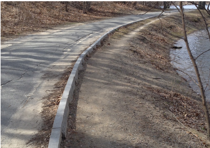
Compaction and erosion from an informal running path behind the curb along the perimeter path below Pinebank.
