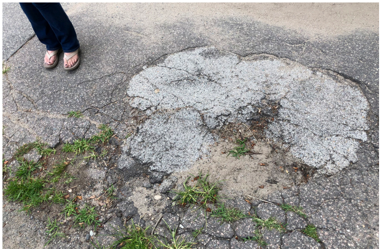
Patched area of bituminous path; Bituminous pavement cracking.
