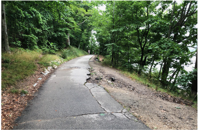
Degraded path edge and resulting erosion.
