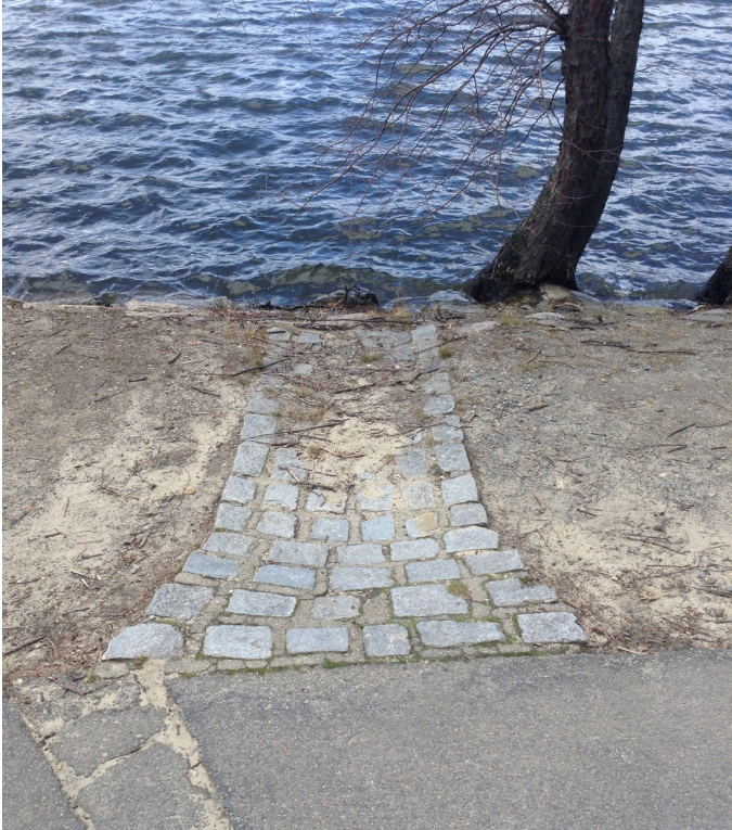
Sediment collecting in cobblestone spillway. Inlets with sediment traps will be retrofit into existing spillways.
