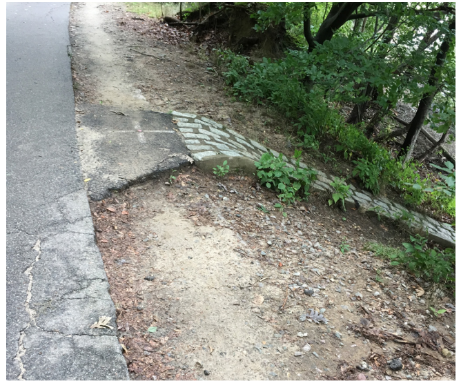
Compaction leaves spillways elevated above the adjacent ground. Water currently flows around the swale, furthering the erosion. A hardened cobble edge will protect the steep slope and direct water to the existing cobblestone spillway.
