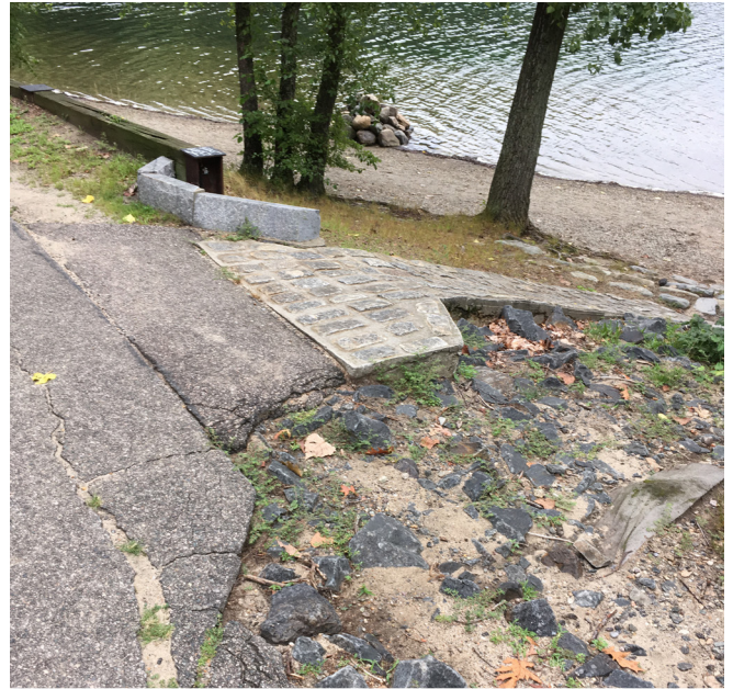
Degraded pavement and erosion around cobblestone spillway. Surface grades will be adjusted to direct water to the spillways, which will be retrofit with sediment traps.
