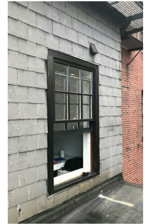
EXISTING FAUX SLATE SIDING TO BE REPLACED
