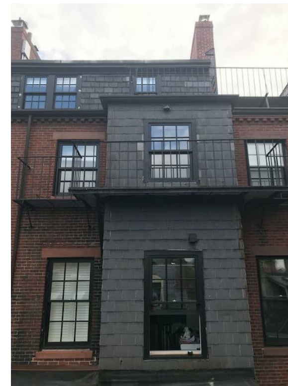
EXISTING FAUX SLATE TO BE REPLACED
