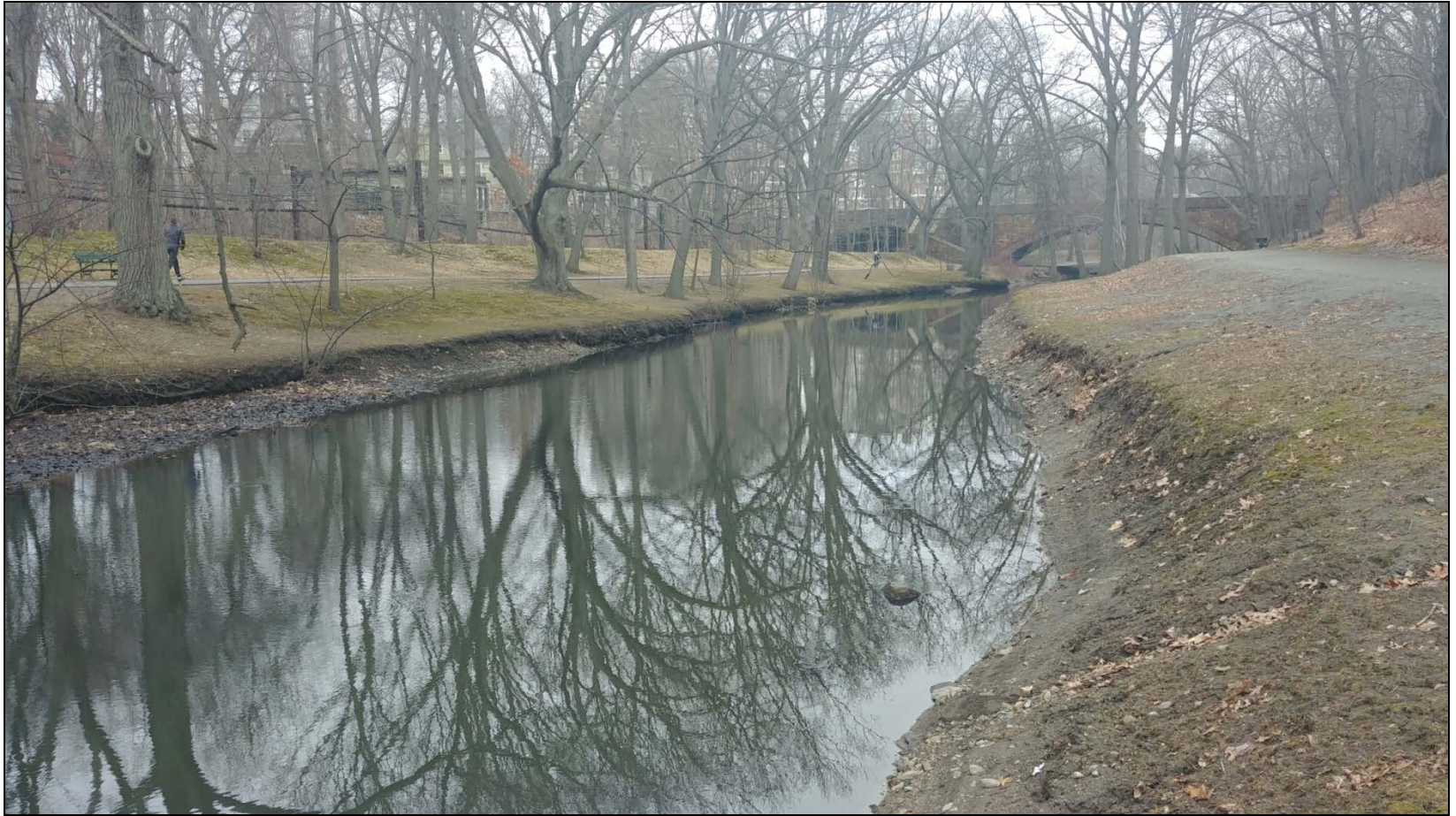
Photograph 7: Eroding stream banks along the Riverway .
