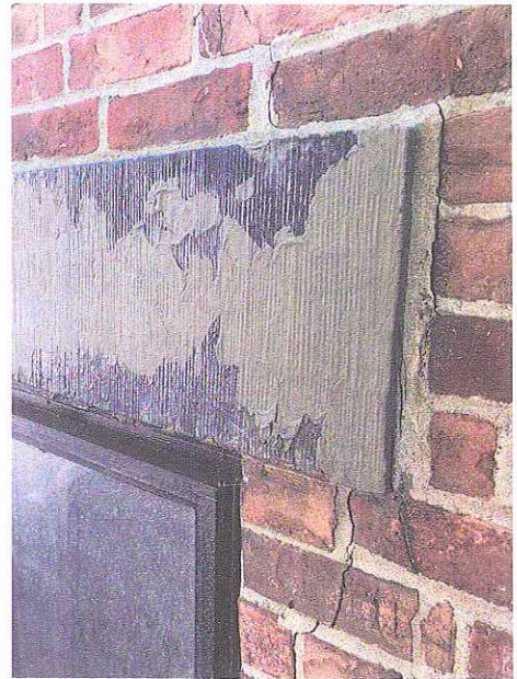
Brownstone Lintel in Good Condition with Two Iterations of Paint (Black & Brown); Re-Set & Replacement Lintels to be Unpainted
