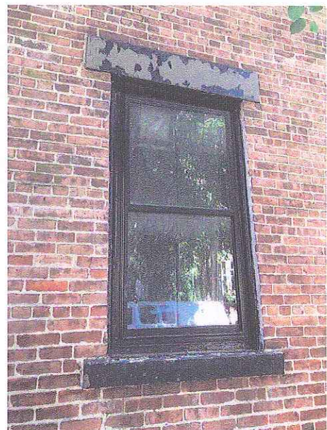
Second of Two 2-over-2 Sash on Brimmer Street Facade; Sash to be Repaired; Frame & Storm Window Replaced; Brownstone Sill & Lintel to be Re-Set and Paint Removed
