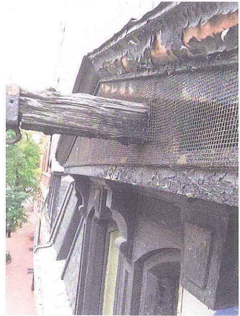
Deteriorated Hayloft Timber to be Replicated; Painted Metal Bird Screening to be Replaced with More Subtle Nylon Mesh Recessed into Gable
