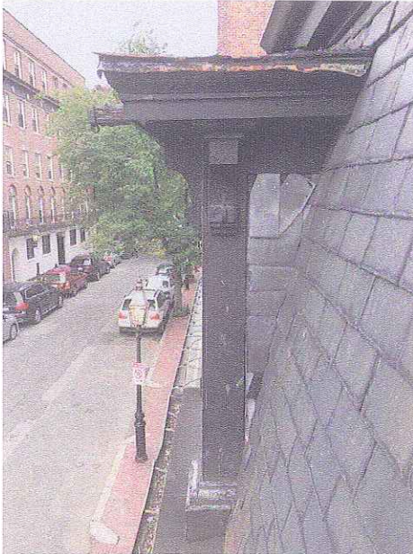
Looking West at Mansard to Gable Roofed Dormer Shared with Neighboring Twin Property; Disrupted Slates on Sidewall & Rusting Metal Roof
