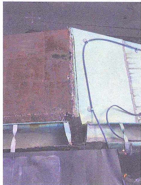
Abutter's Copper Roof at Gable Dormer to Right; 57 Brimmer's Rusted Metal Roofing at Left
