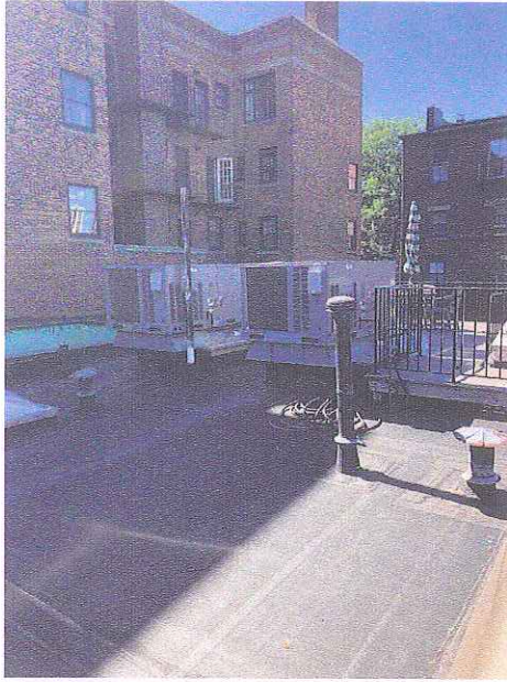
Air Handlers & Roof Deck on Adjacent Property
