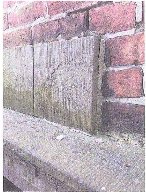
Brownstone Lintel Above Hooded Entrance Lintel; Deteriorated Two-Piece Lintel to be Replaced
