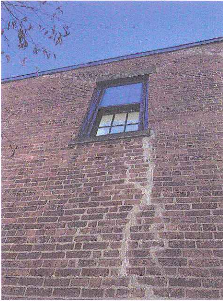
Vertical Cracks in Brimmer Street Facade; Damage was Prior to Foundation Repairs
