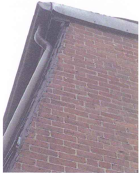
Southeast Corner Showing Transition from Mansard Roof Slope to Adjacent Brick; Roofing Cement to be Removed and Copper Flashing to be Installed
