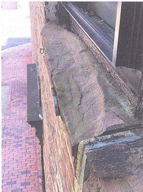
Severely Deteriorated Brownstone Sill at Second Floor
