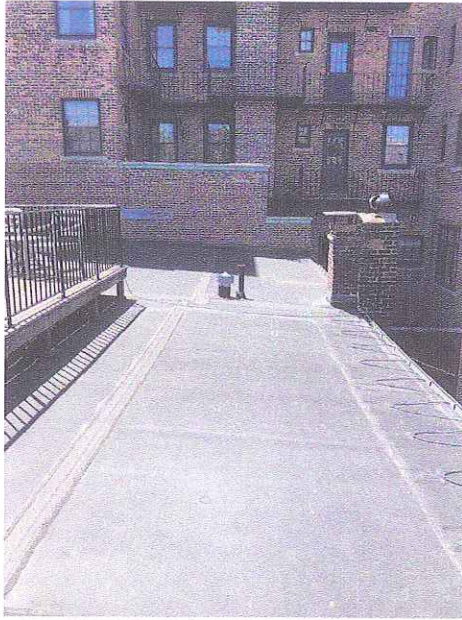
Looking West From Back Edge of Roof; Three Adjacent Properties with Same Roof Slope with Five-Story Brick Building Beyond
