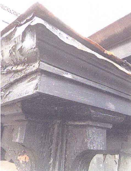
Wood Cornice, Rake, Fascia & Brackets; Rusted Metal Roofing to be Replaced in Copper to Match Profiles
