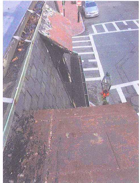
Aerial View of Rusted Metal Roofing at Gable (Foreground) and Shed (Background) Dormers
