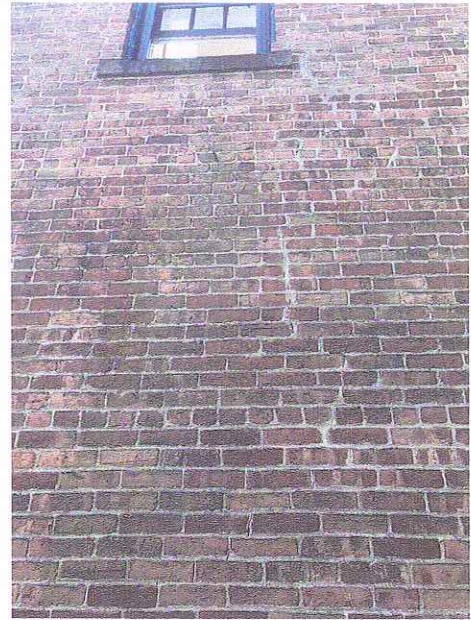
Smaller Vertical Cracks on Brimmer Street; Repairs and Repointing to be Performed Followed by Gentle Masonry Restoration Cleaning
