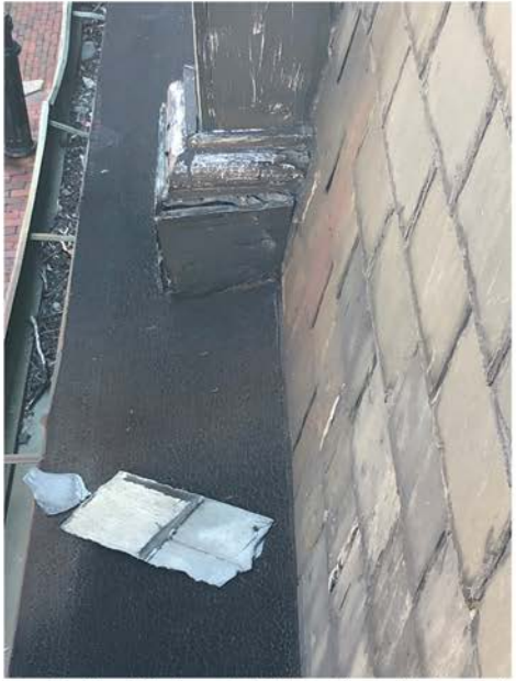
Loose, Fallen Slate on Roll Roofing at Eave Flare; Slates to be Replaced & Eave to be Copper
