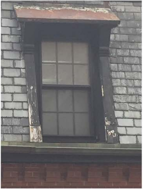
Shed Dormer on Chestnut Street Facade; Sash & Frame to be Retained; Storm Window to be Replaced; Wood Surround to be Repaired; Rusted Metal Roof to be Replaced
