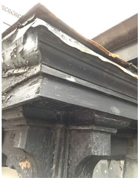
Wood Cornice, Rake, Fascia & Brackets; Rusted Metal Roofing to be Replaced in Copper to Match Profiles
