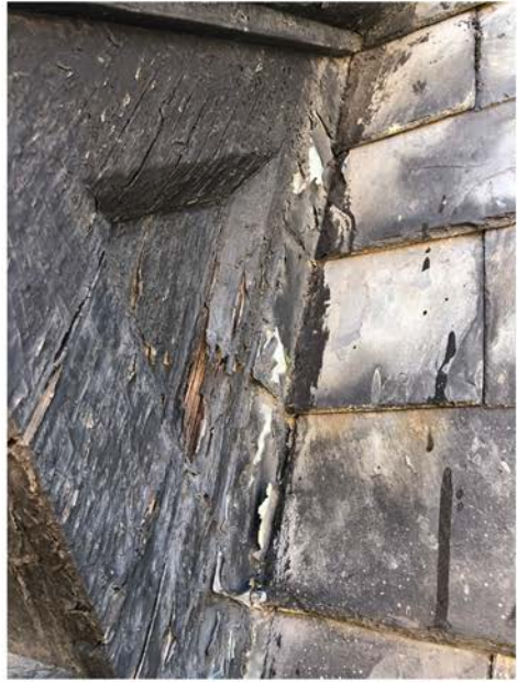
Side of Bracket at Shed Dormer with Roofing Cement to Slated Mansard; Wood to be Restored and Copper Step Flashing to be Provided to Dormer Woodwork
