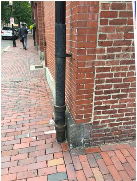
Southeast Corner at Brimmer & Chestnut Street; Front Facade Bricks Differs from Side Facade Bricks
