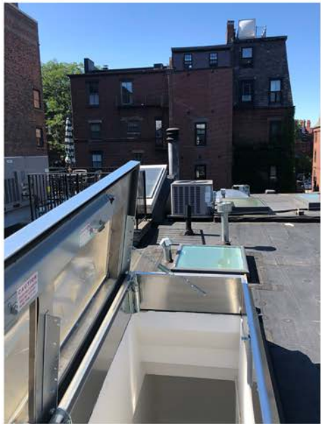
Skylight Roof Hatch at 57 Brimmer Street; Six-Story Building Beyond on Otis Street
