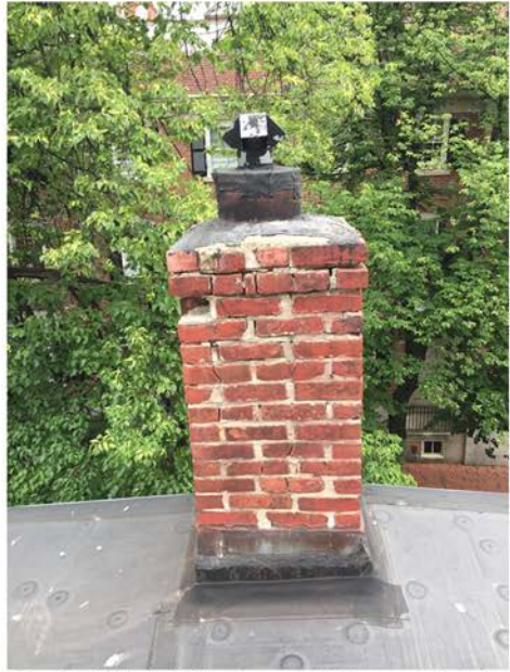
Central Main Chimney on Brimmer Street; Dryer Vent to be Removed & Clay Chimney Pot to be Installed in its Place; Upper Portion to be Rebuilt
