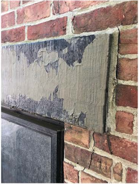
Brownstone Lintel in Good Condition with Two Iterations of Paint (Black & Brown); Re-Set & Replacement Lintels to be Unpainted
