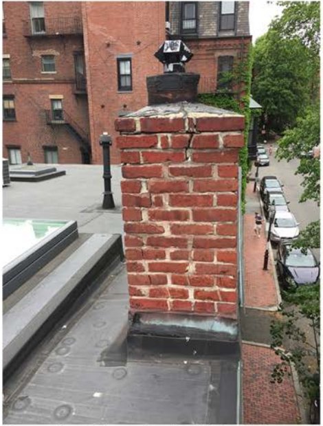
Reconstruct Upper Part of Main Chimney & Replace Dryer Vent with Chimney Pot
