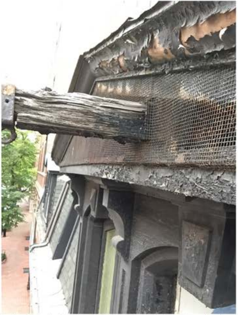
Deteriorated Hayloft Timber to be Replicated; Painted Metal Bird Screening to be Replaced with More Subtle Nylon Mesh Recessed into Gable
