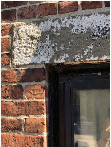
Replacement Granite Lintel on North Facade of Second Floor to be Reused and Painted to Match Color of Brownstone
