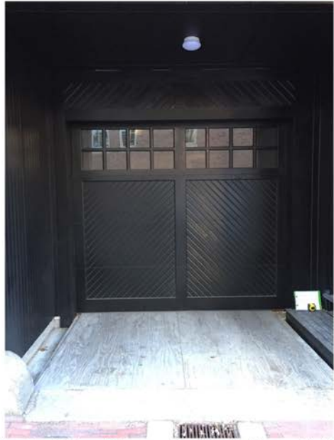
Chestnut Street Garage Door with Upper Lights; Plywood Floor Infill to be Removed for Brick Pavers; No Other Changes to Door & Surround
