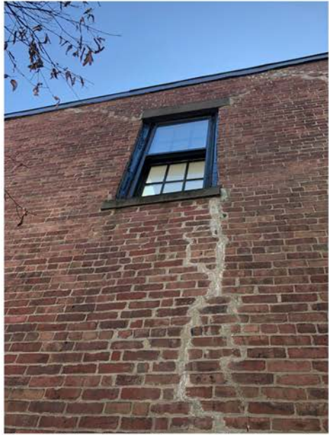
Vertical Cracks in Brimmer Street Facade; Damage was Prior to Foundation Repairs
