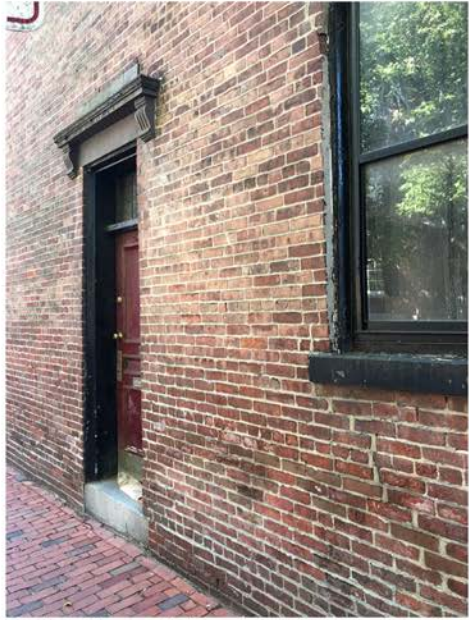
Historic Primary Entrance at 57 Brimmer Street; Tall 12" High Granite Stoop Up from Sidewalk
