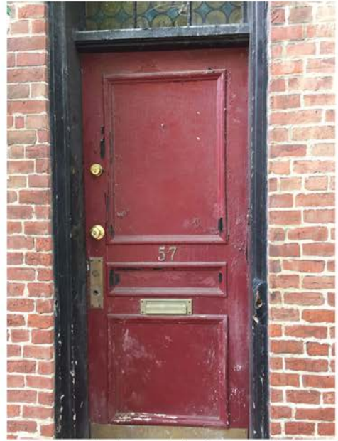
Contemporary Hardware to be Removed; Door to be Patched, Painted & Fixed in Place; Will not be Used as an Entrance or Exit for the School
