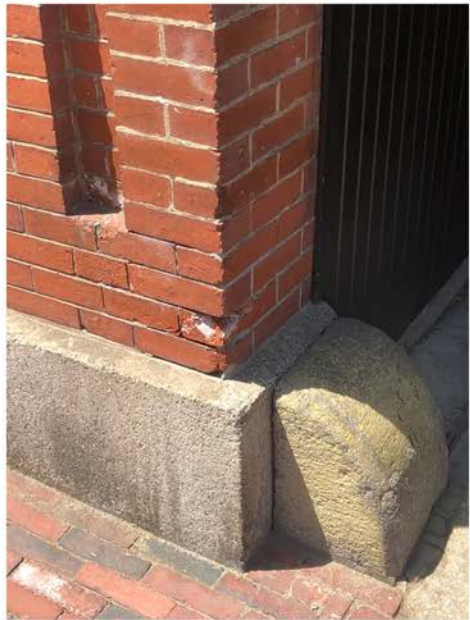
Chipped Brick at Chestnut Street Portico Opening; Granite Plinth and Wheel Guard
