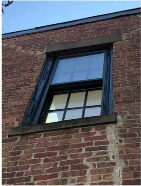
Second Floor Windows are 6-over-6 True-Divided Lights; Sash to be Reused; Frames & Storms to be Replaced; Brownstone Lintels & Sills in Good Condition to be Re-Set, or Replaced in Locations Where Severely Deteriorated
