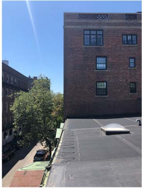
Looking West From Front Edge of Roof; Three Adjacent Properties with Same Roof Slope with Five-Story Brick Building Beyond
