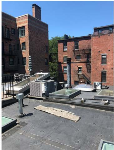
57 Brimmer Street Air-Cooled Condensing Unit; Skylight Hatch & Flue Beyond on Adjacent Property; Five Story Brick Buildings Beyond
