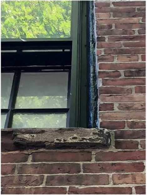
Severely Deteriorated Brownstone Window Sill; Wood Sills and Frames Also in Poor Condition; Replacements to Match Profiles, Colors & Materials
