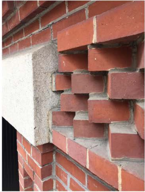
Rotated Bricks in Band Adjacent to Granite Lintel
