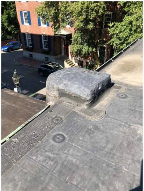
Remnant of Removed Chimney at North Facade; Missing Upper Portion to be Reconstructed with Metal Cap to Match Other Secondary Chimney
