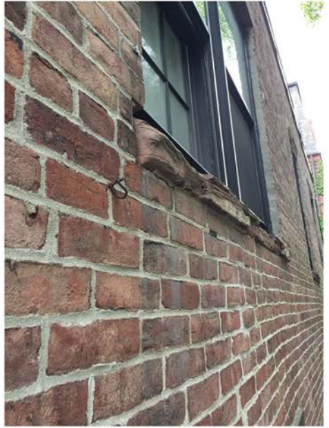
Deteriorated Brownstone Sills to be Replaced
