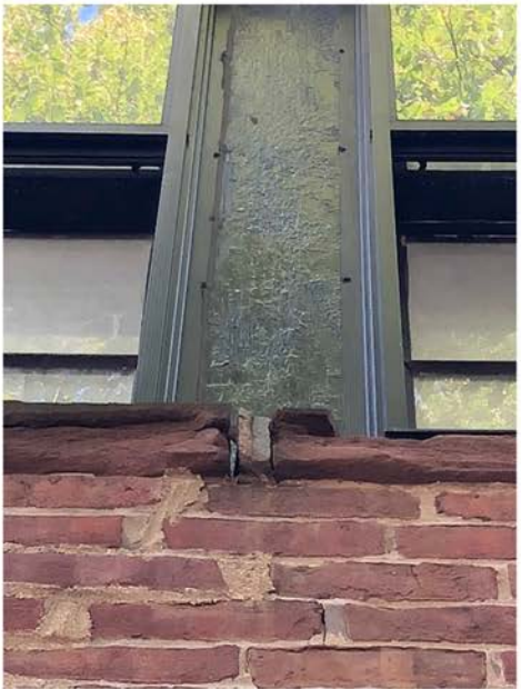
Deteriorated Brownstone Sill at Second Floor Window
