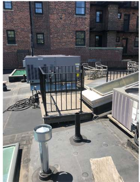
Roof Deck and Air Handlers at Adjacent Building; Brick Building Beyond on Chestnut Street
