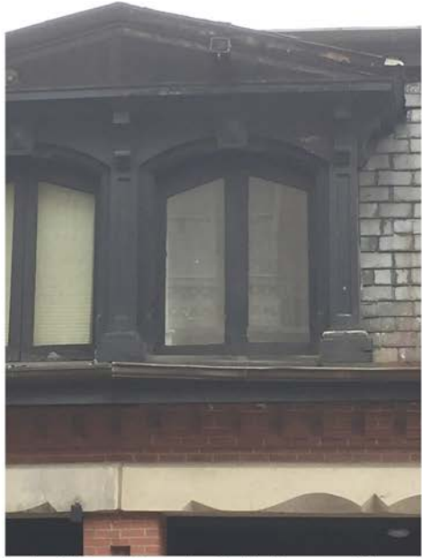
Chestnut Street Facade Gable Dormer Shared by Adjacent Buildings (Right Side is 57 Brimmer Street Bldg.); In-Swing Casement Window to be Repaired
