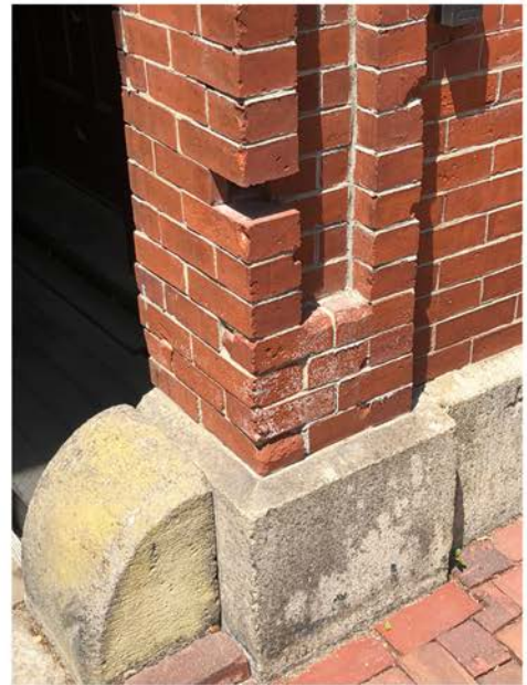
Missing & Chipped Bricks at Chestnut Street Portico; Granite Plinth and Wheel Guard
