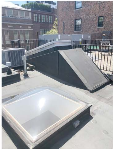
Skylight in Foreground and ACCU at Left on 57 Brimmer Street Building; Raised Hatch, Roof Deck & Air Handlers Beyond on Adjacent Building
