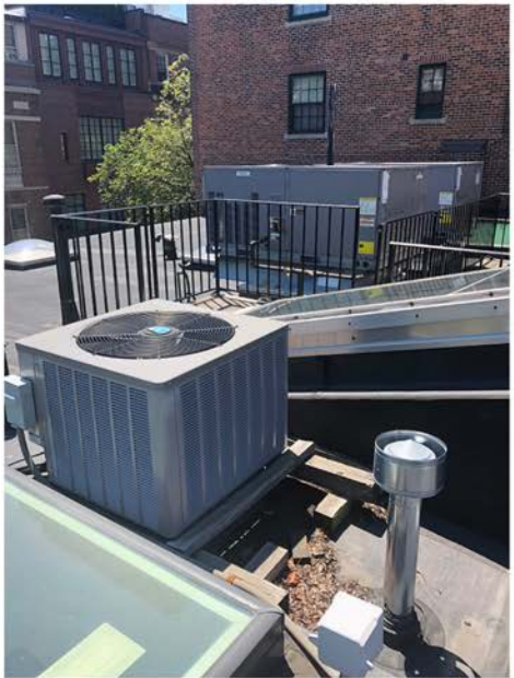
ACCU for 57 Brimmer Street; Air Handlers Beyond on Adjacent Building
