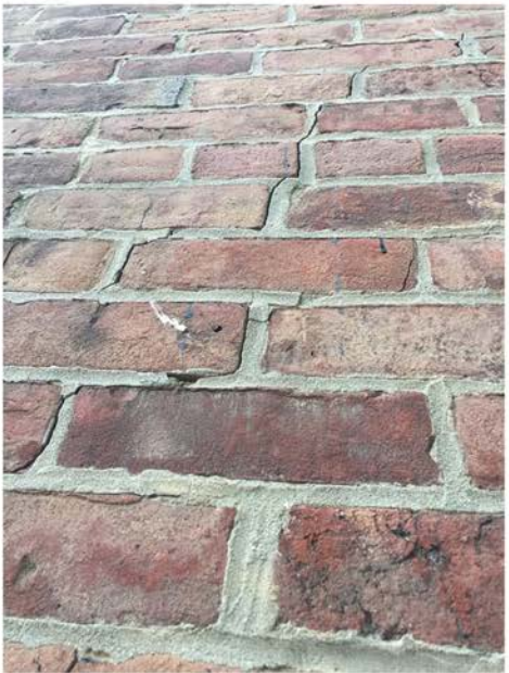
Detail of Brimmer Street Brickwork Showing Former Inappropriate "Scrub Coat" Repointing
