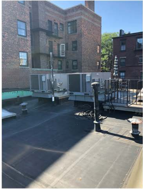
Air Handlers & Roof Deck on Adjacent Property
