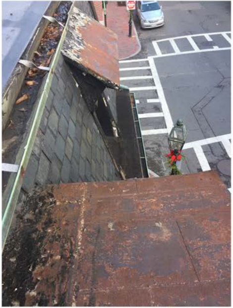
Aerial View of Rusted Metal Roofing at Gable (Foreground) and Shed (Background) Dormers
