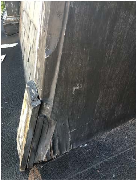
Deteriorated Plywood Jambs at Shed Dormer; Loose Replacement Plinth at Outer Casings; All Carpentry to be Replicated, Flashed & Painted
