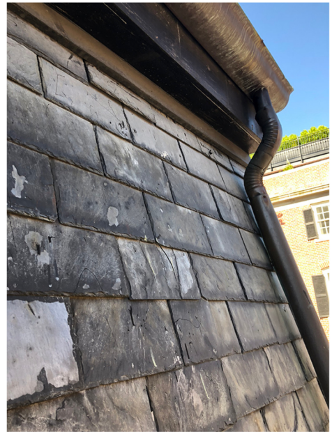
Deteriorated Dark Gray Slate Roof with Copper Gutter, Copper Rain Leader and Painted Wood Fascia
