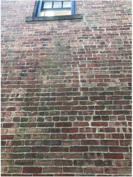
Smaller Vertical Cracks on Brimmer Street; Repairs and Repointing to be Performed Followed by Gentle Masonry Restoration Cleaning
