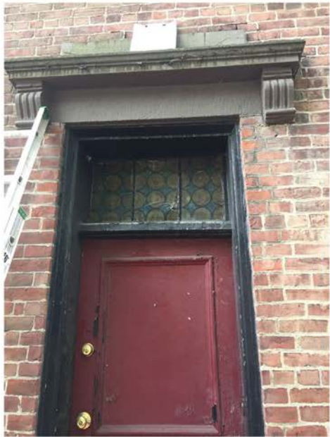
Hooded Stone Lintel and Glass Transom Panel; Door & Transom Frames to be Retained & Painted
