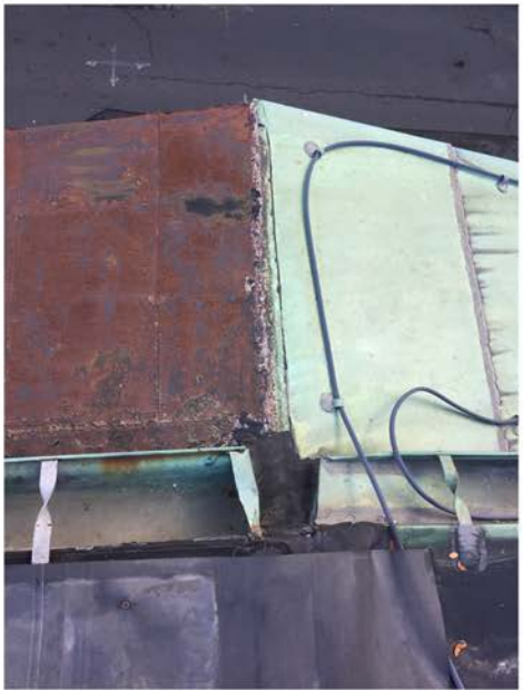
Abutter's Copper Roof at Gable Dormer to Right; 57 Brimmer's Rusted Metal Roofing at Left
