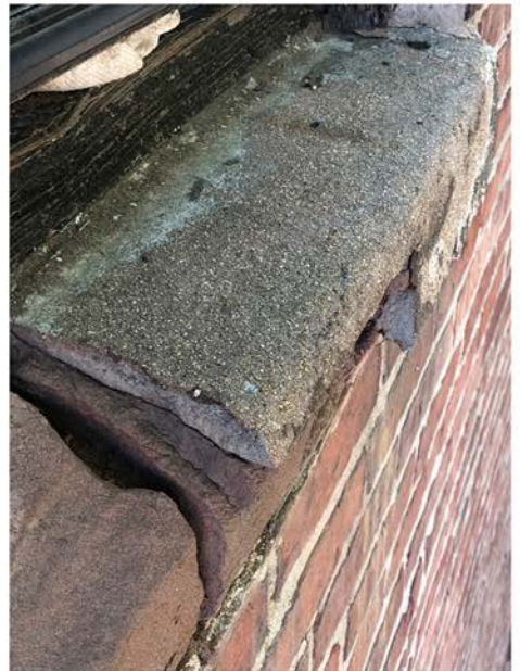
Failing Patch at Severely Deteriorated Brownstone Sill
