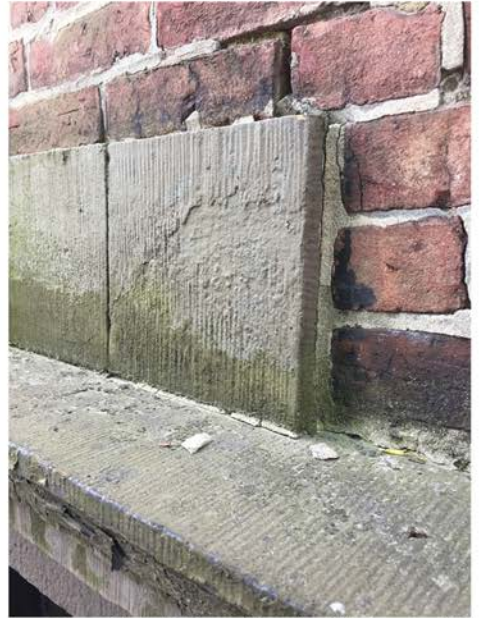
Brownstone Lintel Above Hooded Entrance Lintel; Deteriorated Two-Piece Lintel to be Replaced
