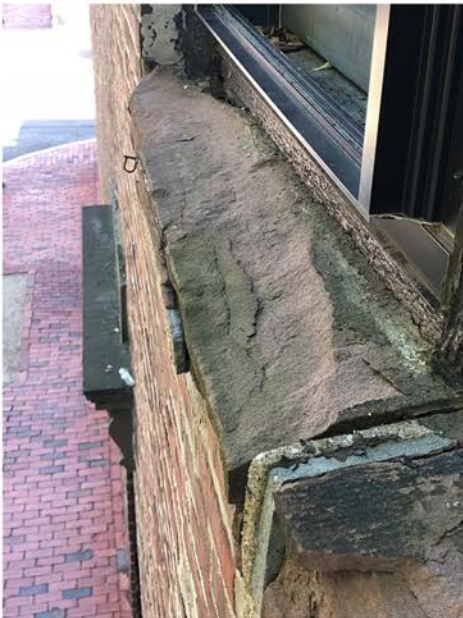
Severely Deteriorated Brownstone Sill at Second Floor
