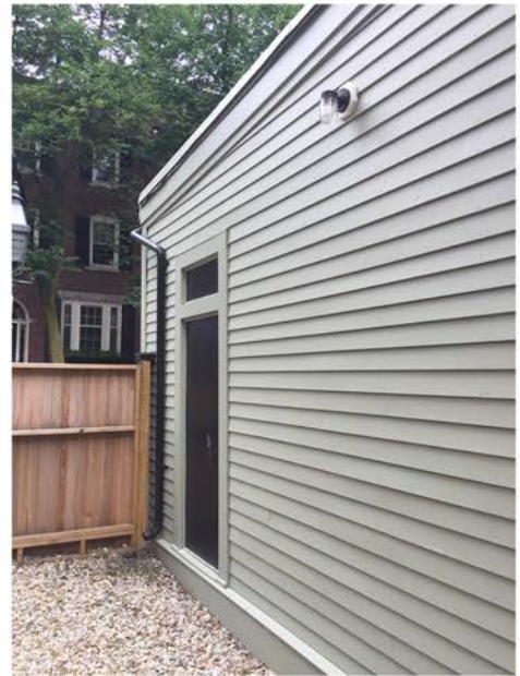
North Elevation of One-Story Garage with Service Door Opening and Transom (No Door or Transom at Present); Door & Transom to be Provided into Rear Yard as Replication of Missing Components
