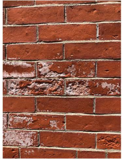
Selective Deteriorated Bricks on Chestnut Street Facade to be Replaced in Kind Where Needed
