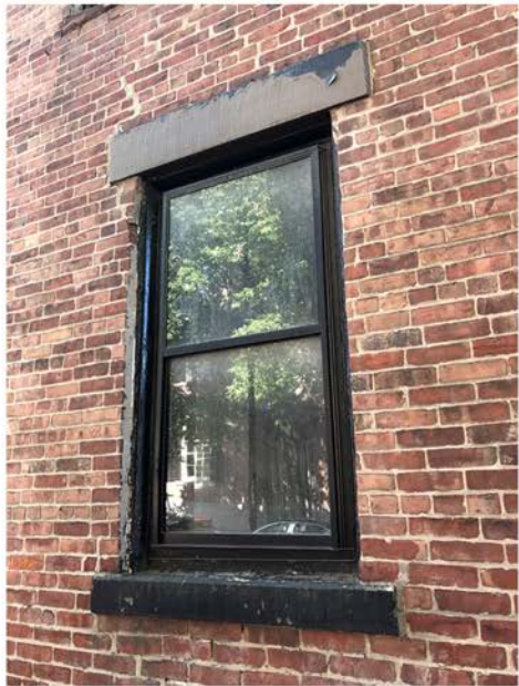
First of Two 2-over-2 Sash on Brimmer Street Facade; Sash to be Repaired; Frame & Storm Window Replaced; Brownstone Sill & Lintel to be Re-Set and Paint Removed
