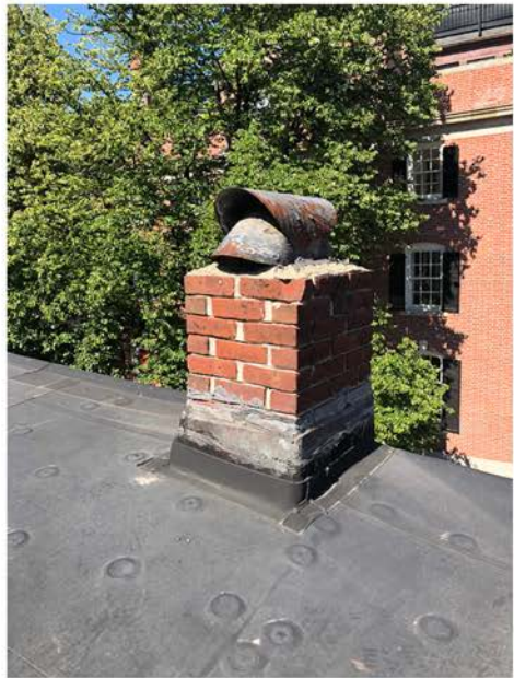
Secondary Chimney on Brimmer Street Near Chestnut Street at SE Corner; Deteriorated Metal Cap to be Replicated in Gray Copper
