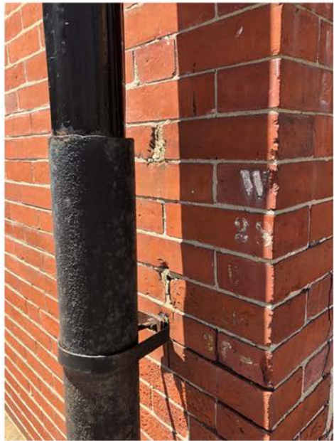
Damaged Bricks at Rain Leader by SE Corner
