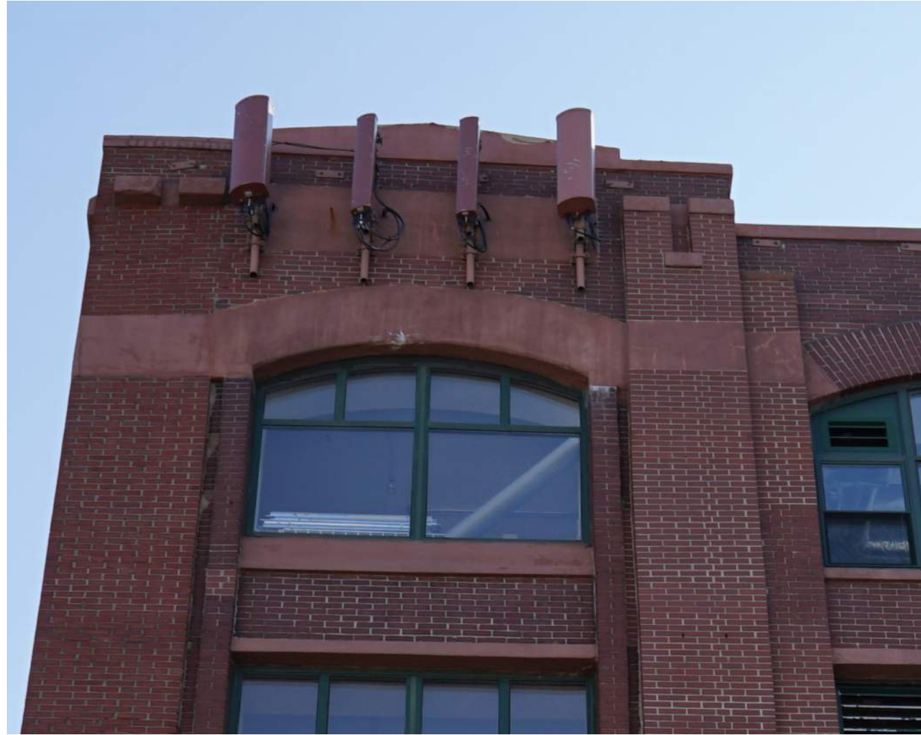
Existing Surface Mounted Cellular Antennas
