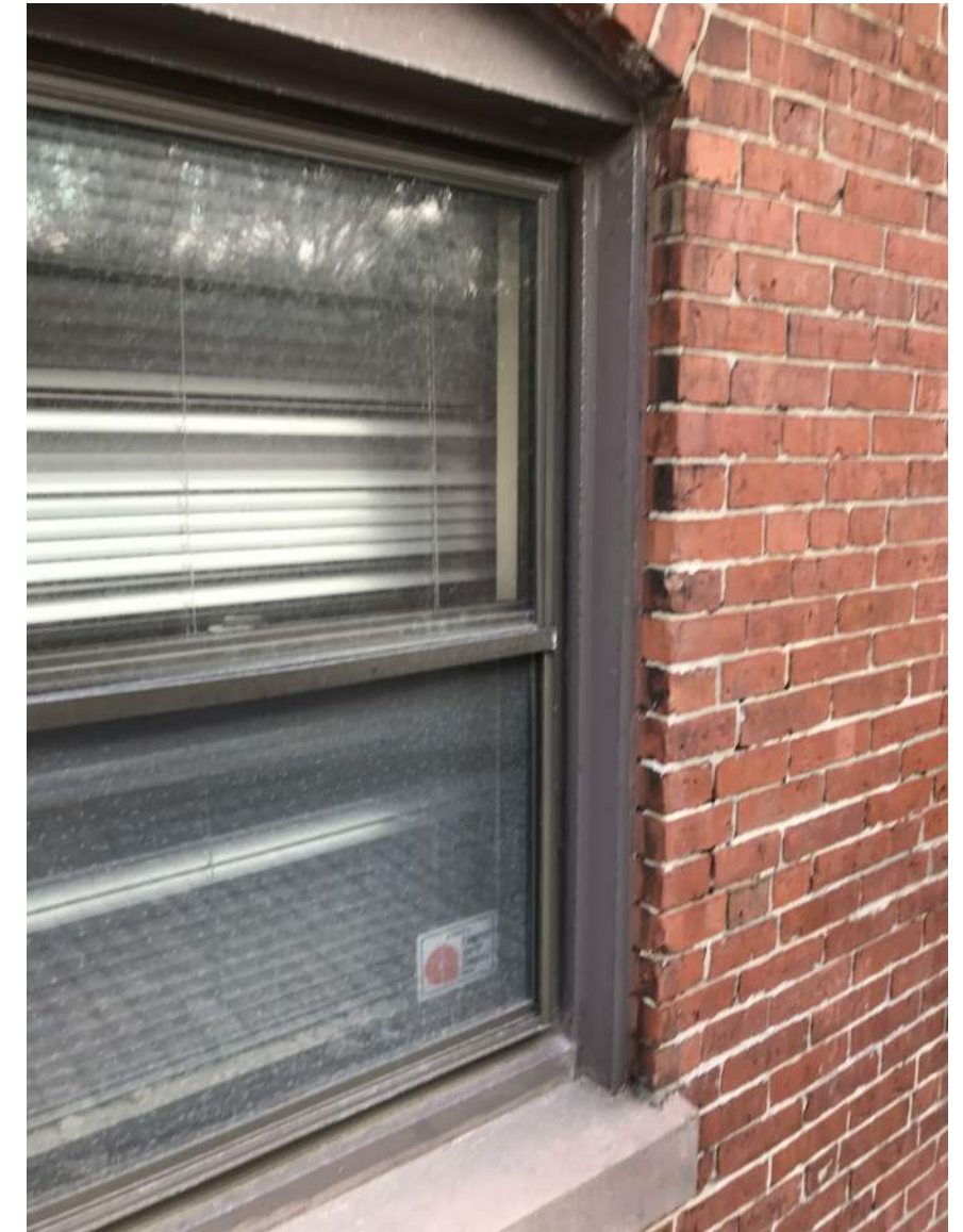
NON-HISTORIC REPLACEMENT WINDOWS AT ALLEY
