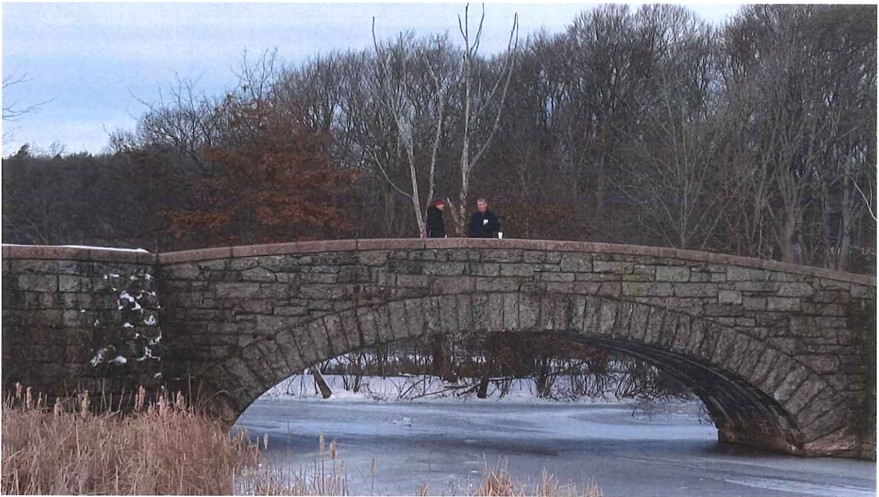
The iconic stone arch bridge. The new cart boardwalk will eliminate golf cart related traffic from this bridge and reestablish the historic bridge to pedestrian only traffic.
