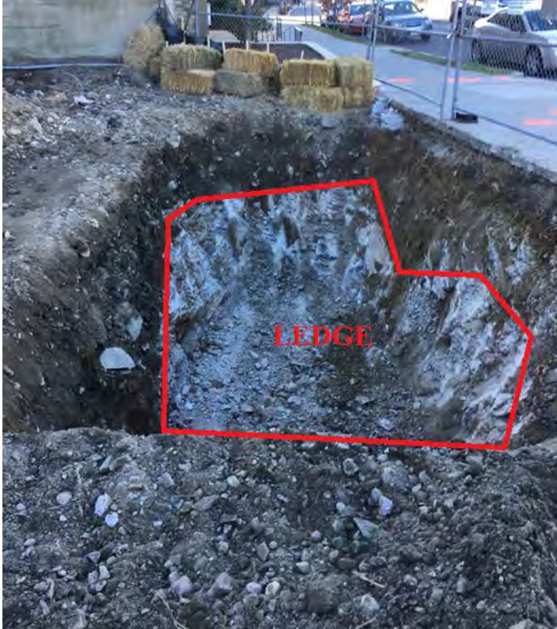
Figure 3 – View of excavation of Drywell #1 and #1B located at the back of sidewalk. A jackhammer was needed to remove between 24-36” of ledge to provide room for the drywells in this area. The proposed trees are approximately 17’ from this area.
