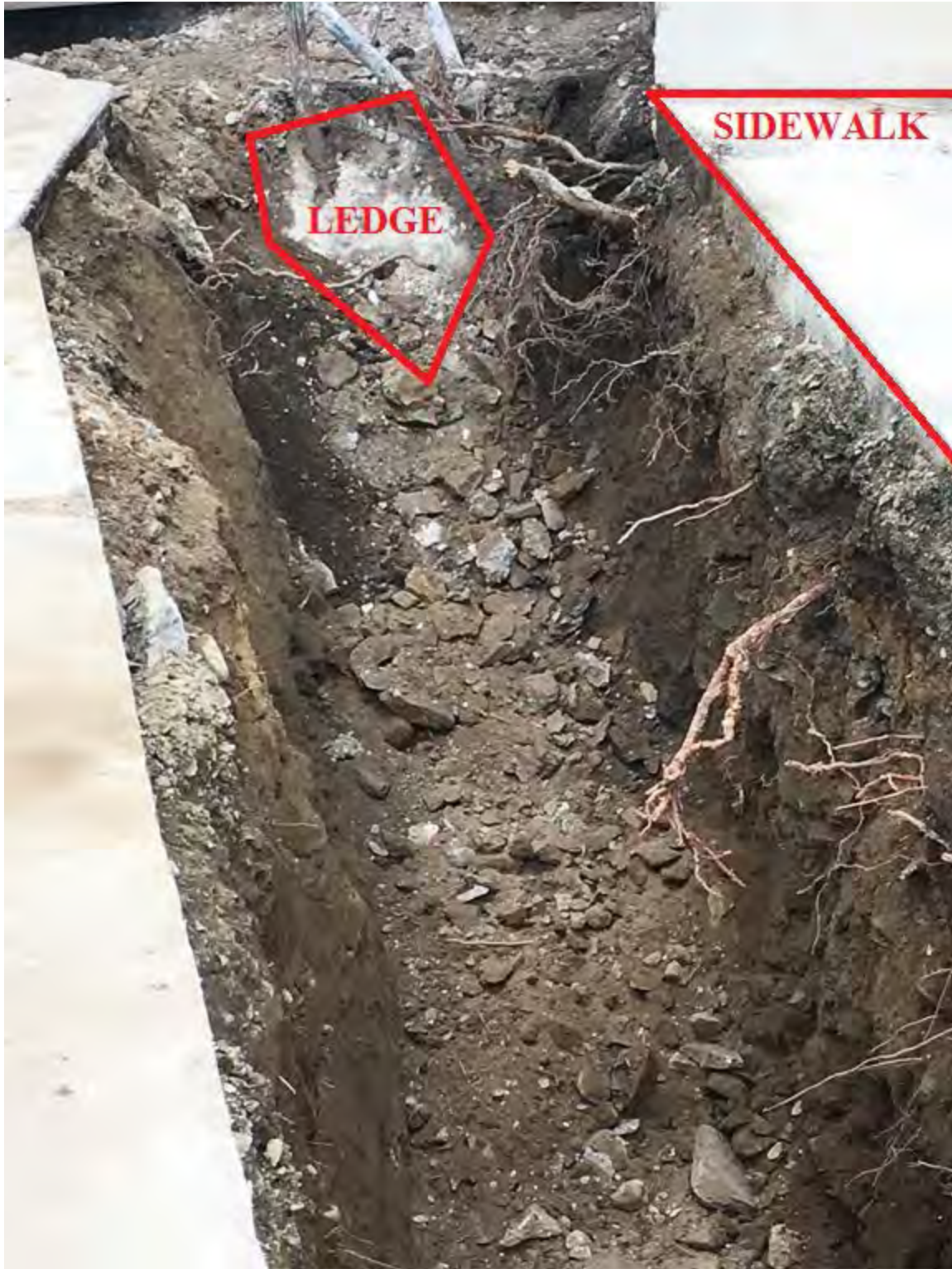
Figure 4 – View of trench for 12” PVC drain line being laid in Commonwealth Avenue (connecting DMH#4 to the drainage infrastructure in Commonwealth Avenue). Ledge is within 12” of the sidewalk in some places.
