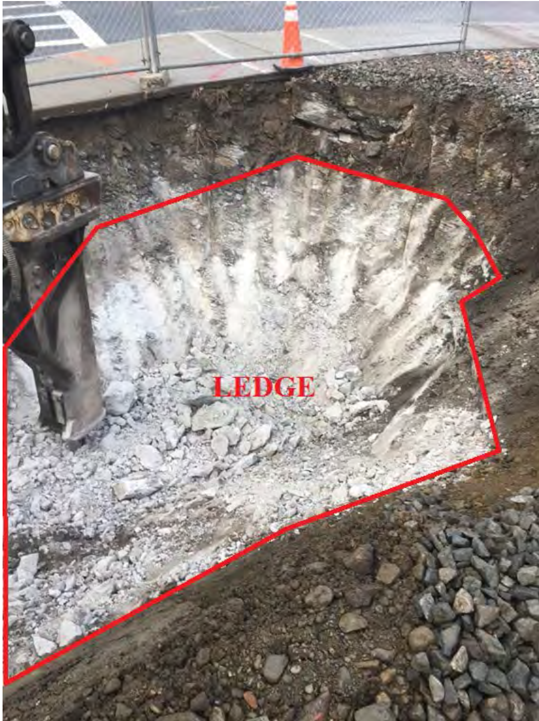
Figure 2 – View of excavation of Drywell #3 and #3B at the back of sidewalk on the corner of Commonwealth Avenue and Mount Hood Street. A jackhammer was needed to remove between 24-36” of ledge to provide room for the drywells in this area. The proposed trees are approximately 20’ from this area.
