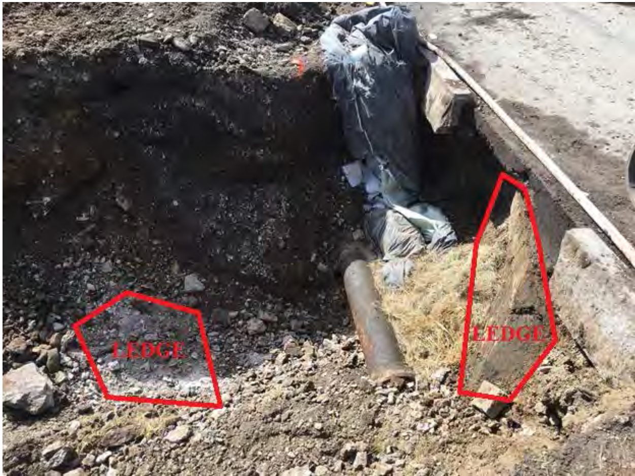
Figure 1 – View of existing 8” water line beneath the existing sidewalk at the fire protection connection point (See Test Pit Locations Plan – Sheet TP-1 for location)
