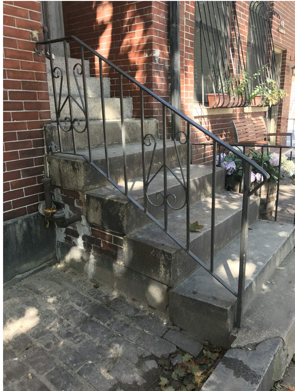
FRONT STOOP TO BE REPAIRED AND RESTORED, AS REQUIRED. STAIR RAILING TO BE REPLACED TO MATCH NEIGHBORING RAILS.
