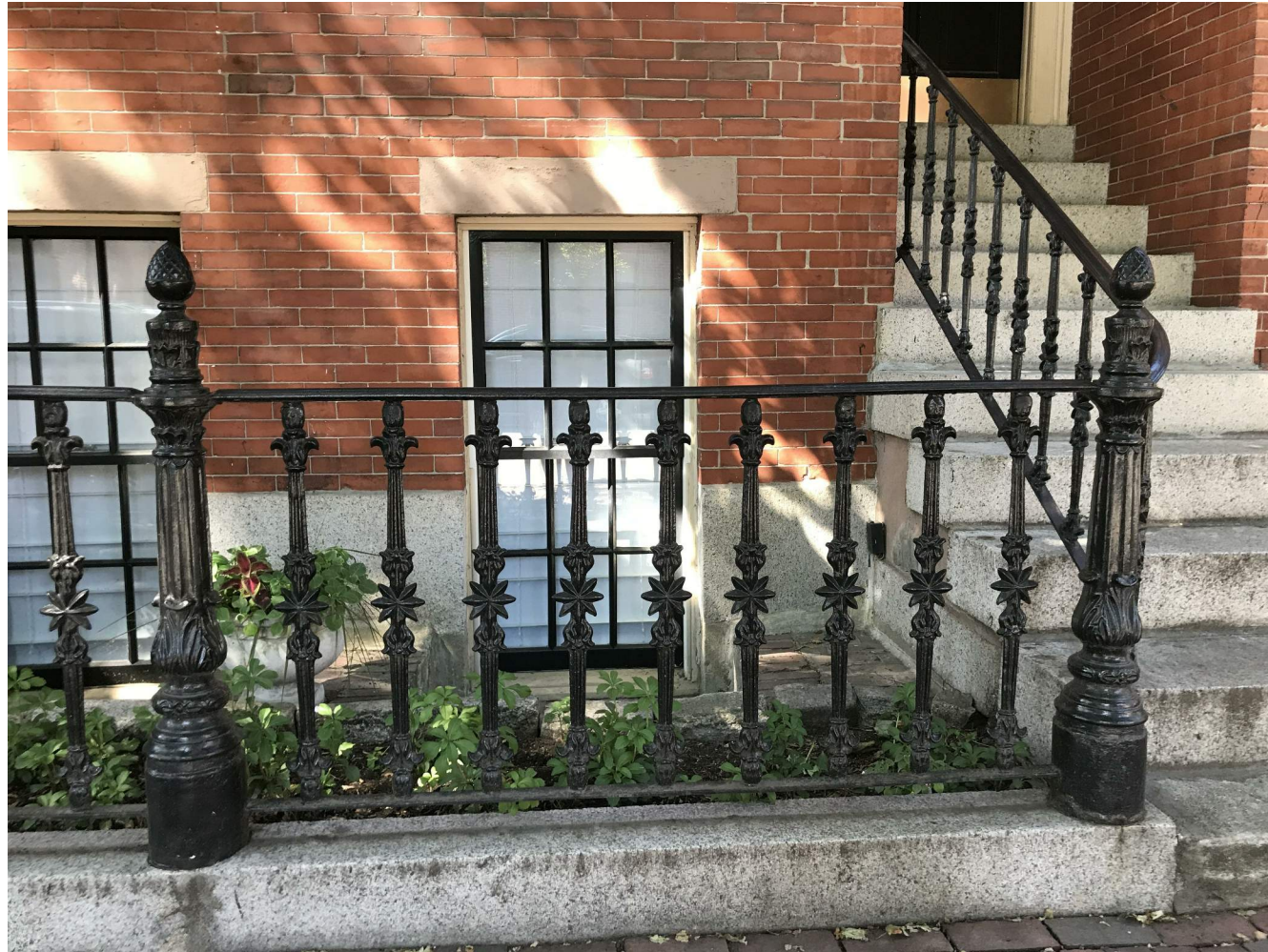
PRECEDENT RAILING - FOUND AT 42/44 CLARENDON ST PROPOSED RAILING TO WRAP UP STOOP STAIR TO MATCH PRECEDENT
