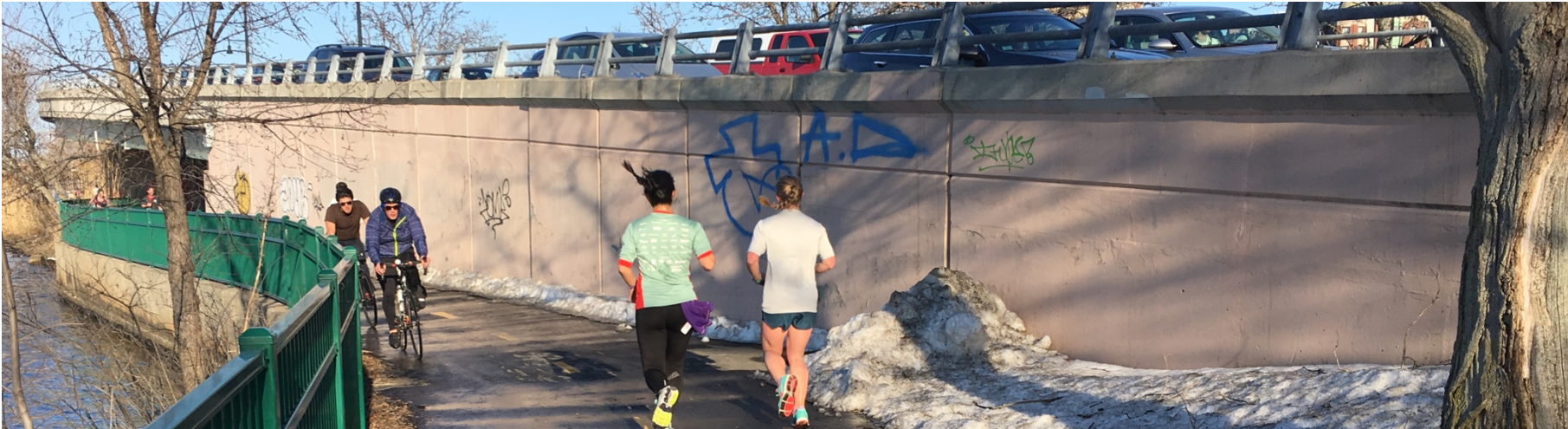
Storrow Drive West ramp wall; photo looking east. Wall is painted pinkish beige and is attractive to graffiti taggers.
