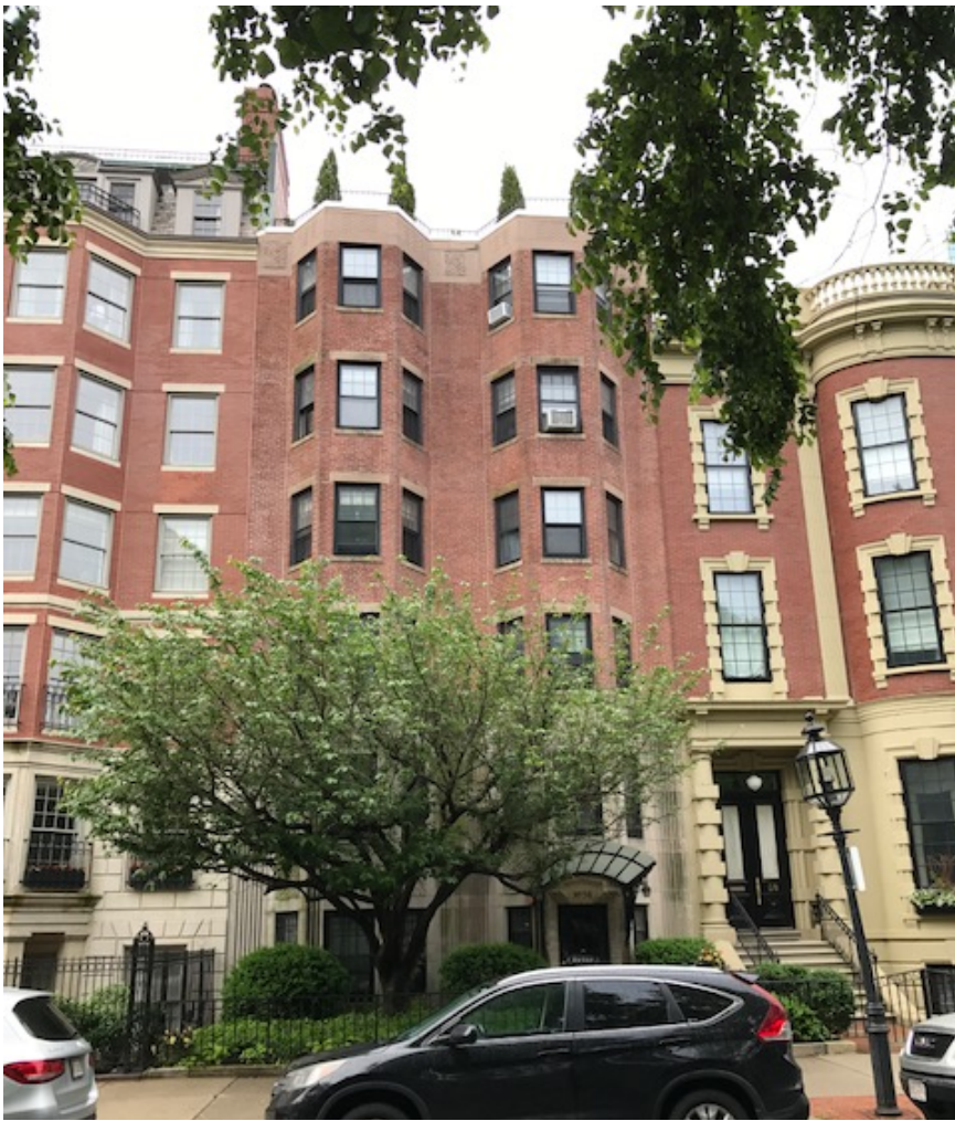
Front of building: No windows affected (Above)
