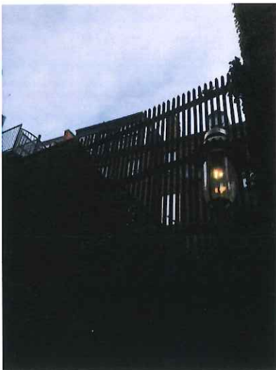
Polygon Window to be replaced, from Alley view
