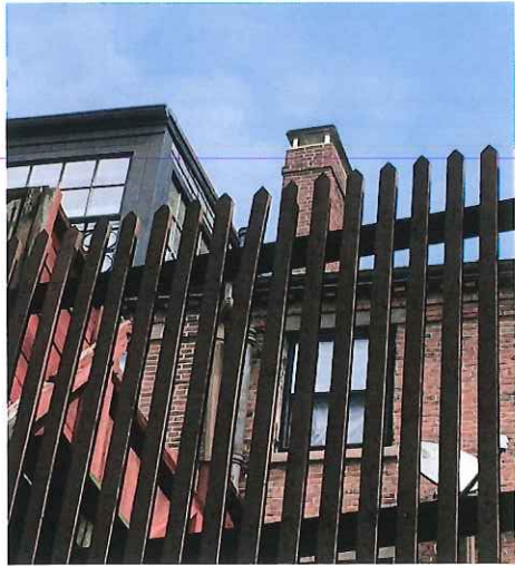
Polygon Window to be replaced, from Alley view
