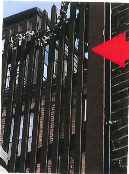
Polygon Window to be replaced, indicated by red arrow. Photo is looking North from Cedar Lane Way.
