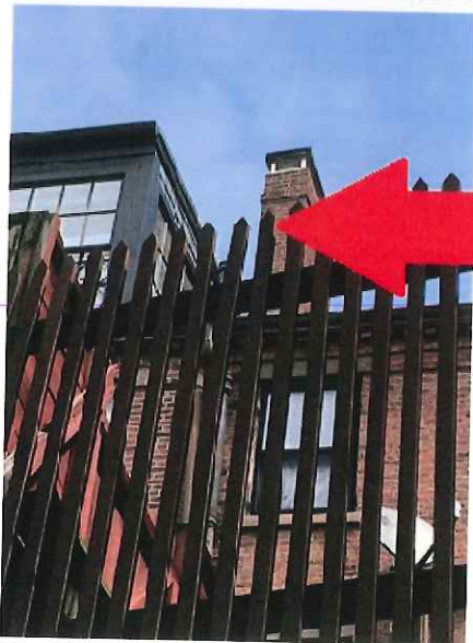
Polygon Window to be replaced, indicated by red arrow. Photo is looking North from Cedar Lane Way.
