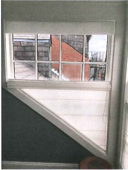
Polygon window to be replaced, interior view.
