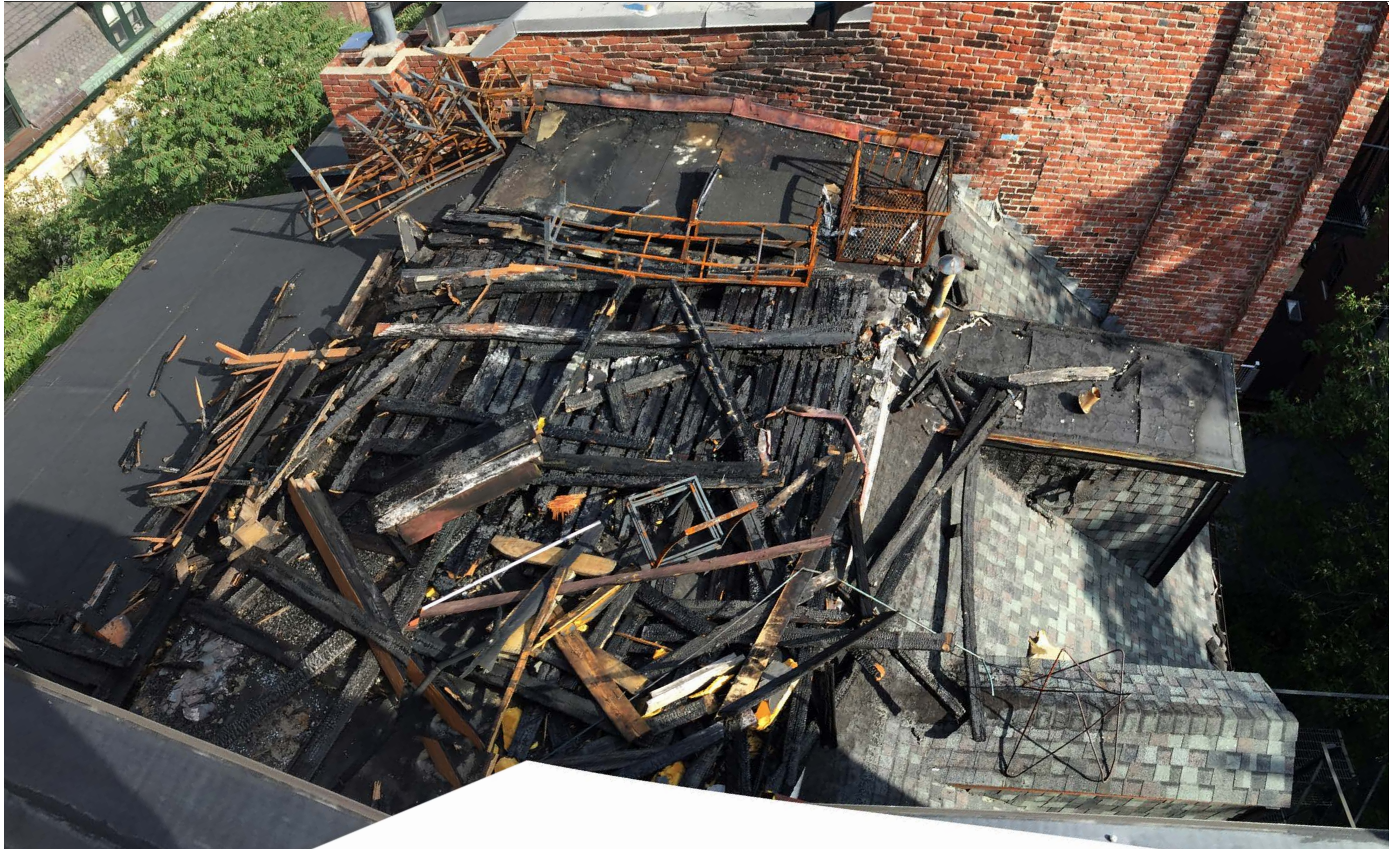
32 Hancock Street Fire Damaged Roof and Deck
