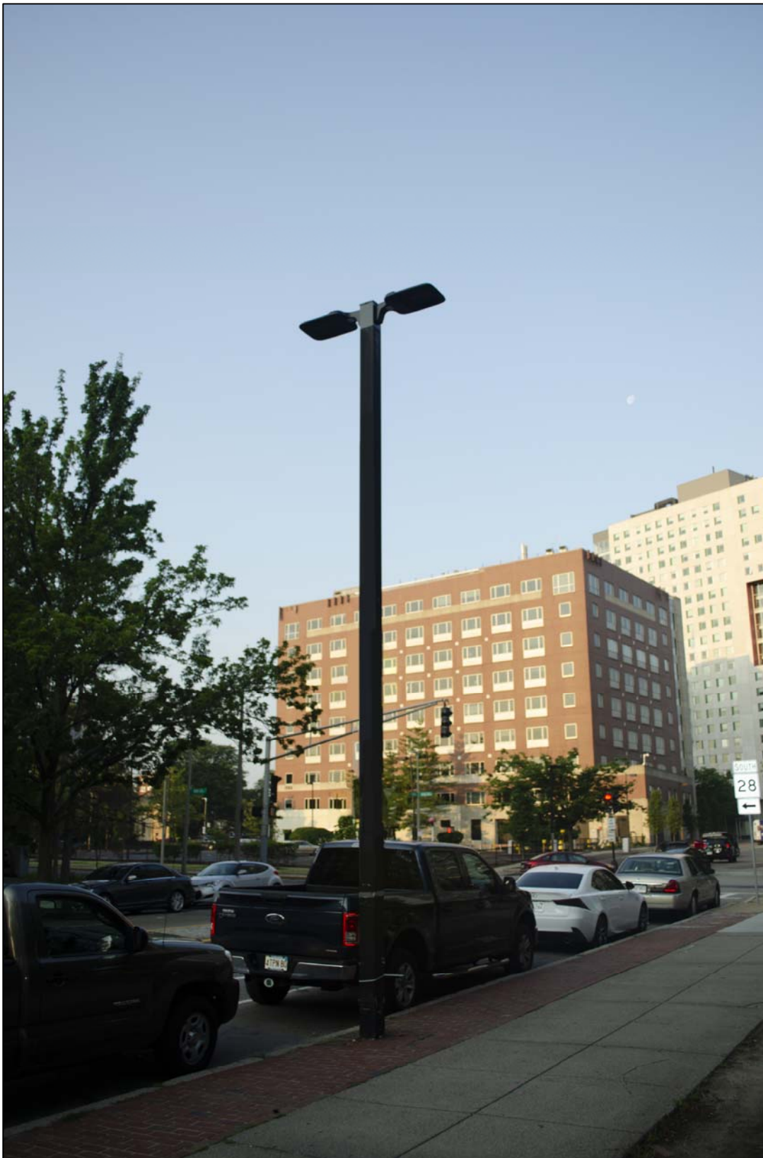
SQUARE CONTEMPORARY LIGHT POLE - DOUBLE AERIATA LUMINAIRE FIXTURE EXISTING CONDITIONS PHOTOGRAPH - EXHIBIT X-2
