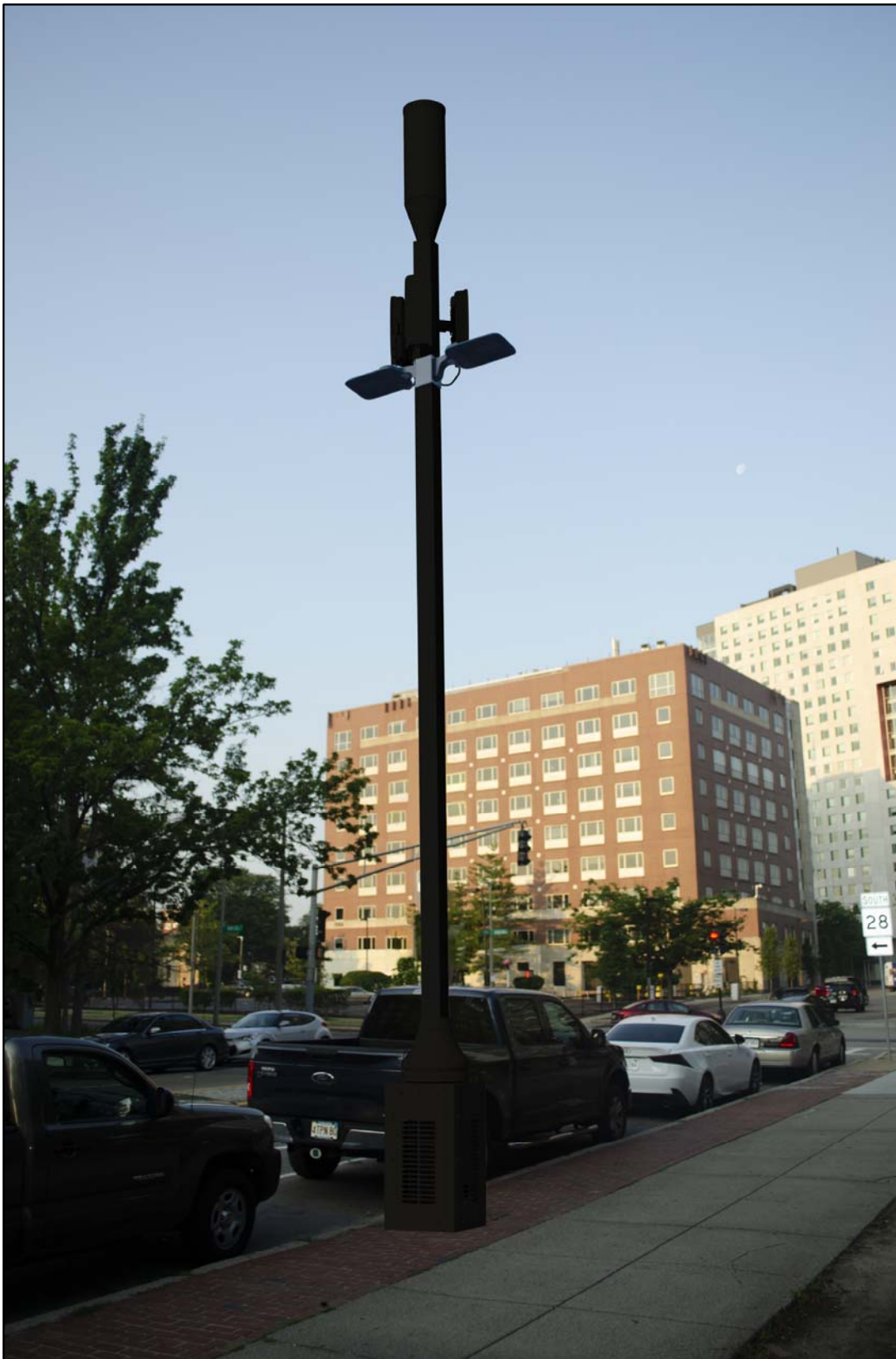
SQUARE CONTEMPORARY LIGHT POLE - DOUBLE AERIATA LUMINARY FIXTURE PROPOSED PHOTOSIMULATION - EXHIBIT X-2A
