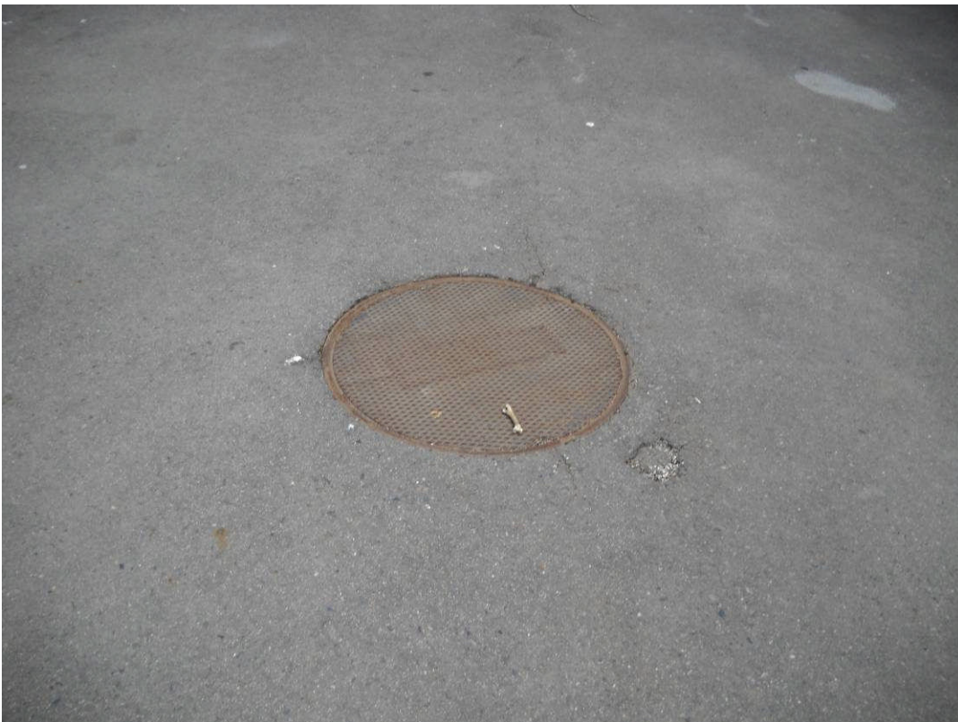
Photograph No. 4: Oil-Water Separator Manhole
