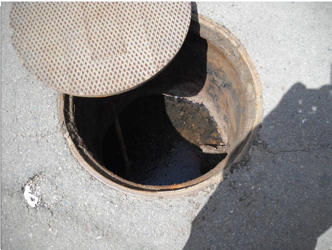
Photograph No. 10: Oil-Water Separator (opened)
