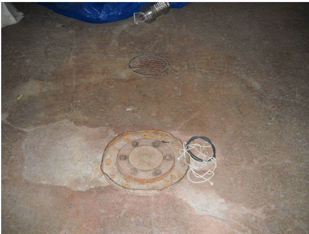
Photograph No. 6: Hydraulic Lift Base
