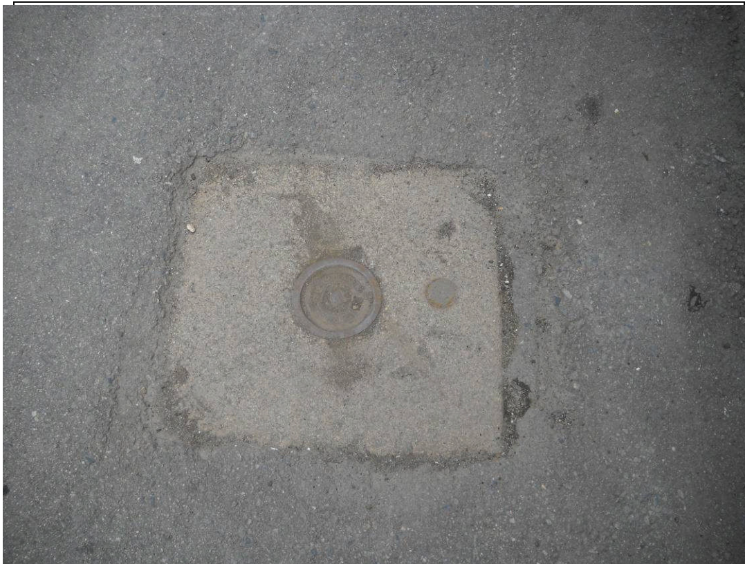
Photograph No. 5: Six-inch UST Fill Port
